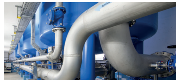
Booster systems, drinking water pumping stations, pressure maintenance
