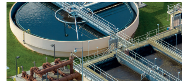
Wastewater pumping stations, pressure maintenance
