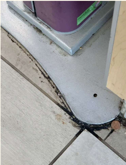
Dirt and black substance on the floor and equipment in the Emergency Room at Sunrise
