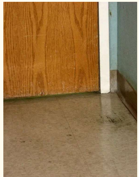
Dirty, moldy floor, wall and doorway in a patient room.
