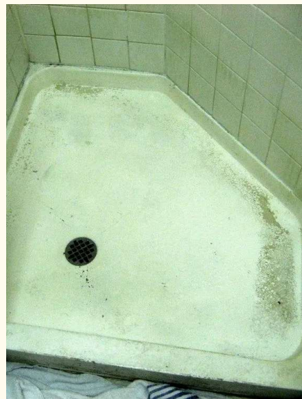
Dirty, worn out shower in a patient room.
