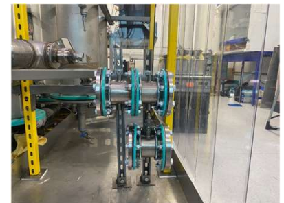
Level control vessels for the reclaimer
