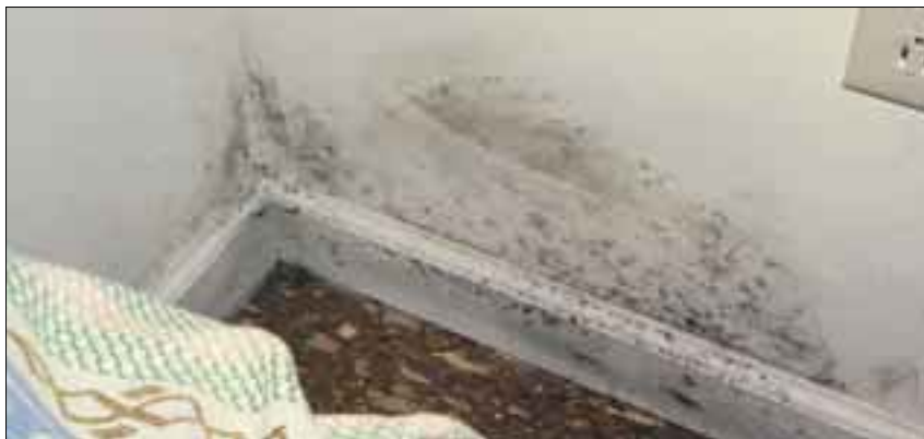
Water infiltration in basements can be a major source of mold in homes. Controlling rain-water and ground-water entry are keys to controlling mold.
