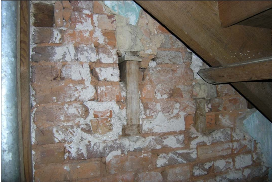
Figure 19. Exposed brick work underneath the stairwell.
