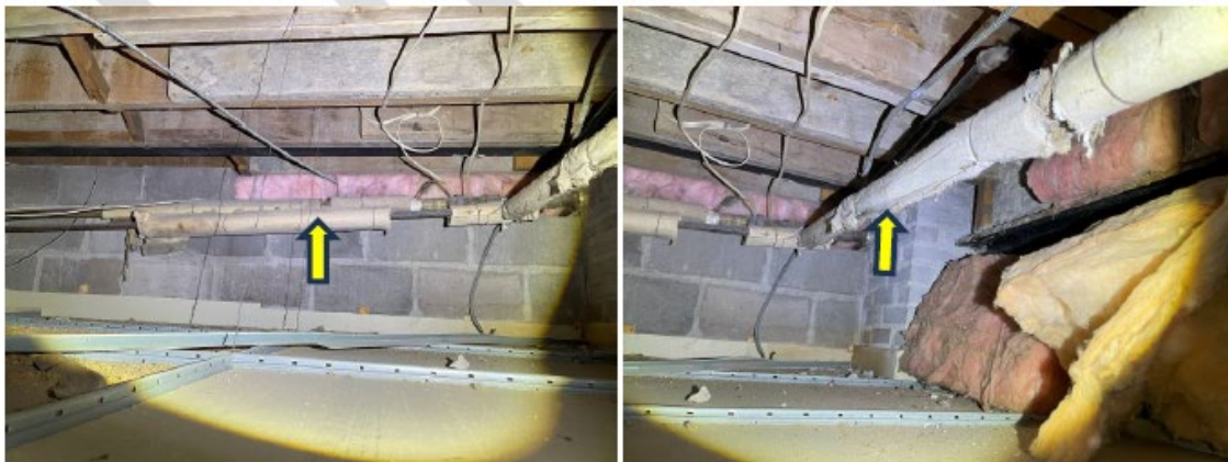
Photograph No. 3.1 and 3.2: View of asbestos-containing pipe straight insulation (tar felt, insulation, wrap) was identified within the west office on the 1st floor municipal office of the subject building.
