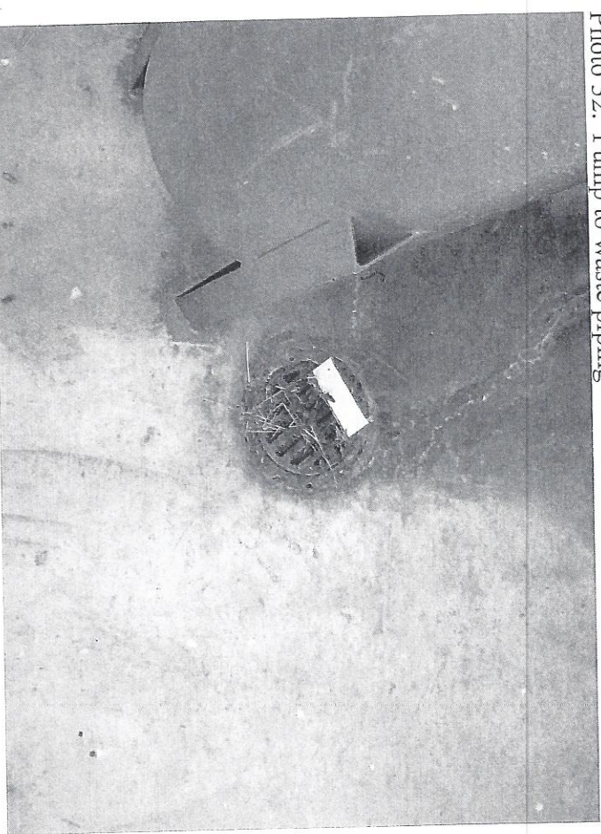
Photo 34. Floor drain in pump house
