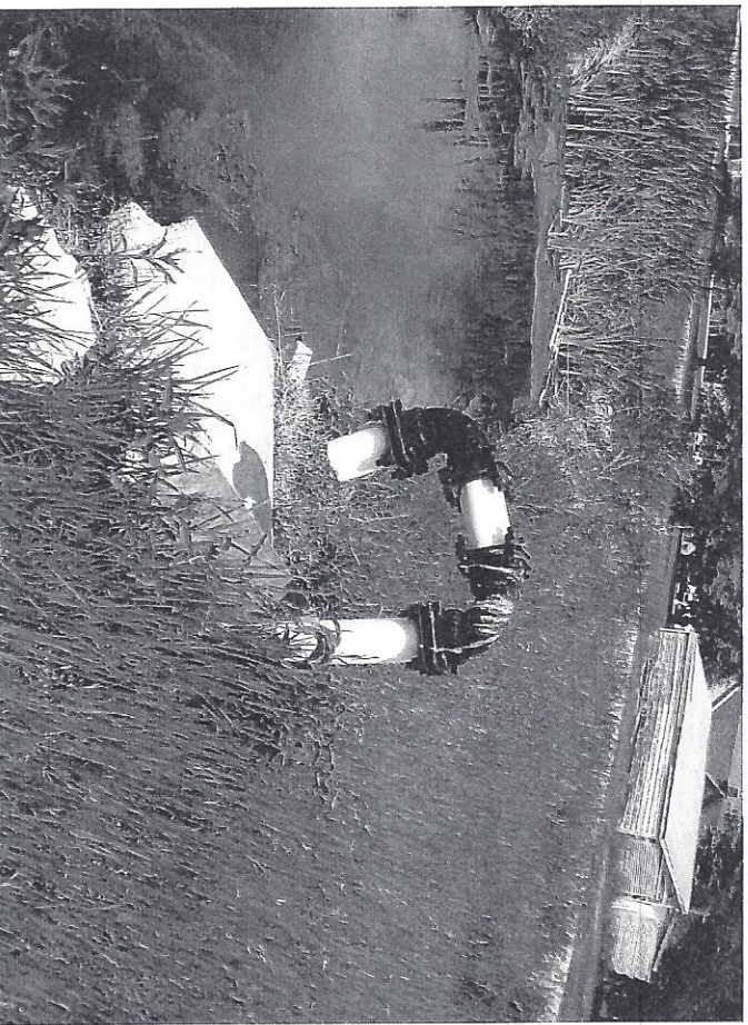
Photo 26. Well #1 pump to waste discharge
