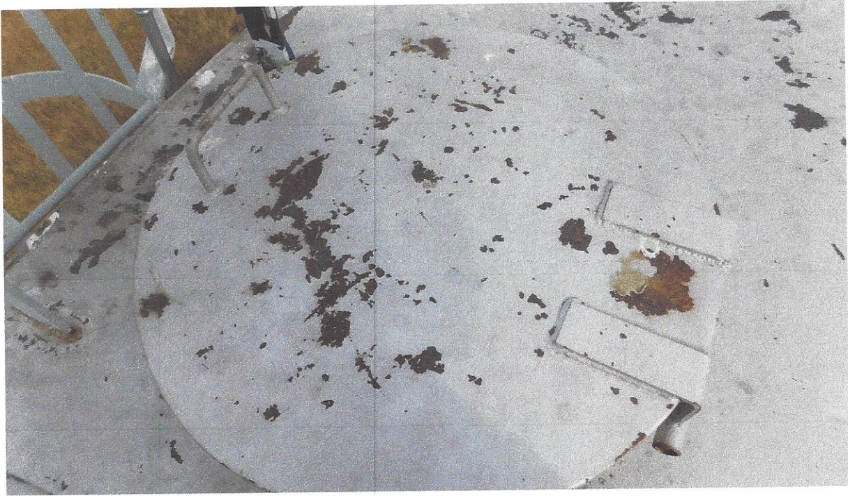
11.) Primary Roof Hatch
