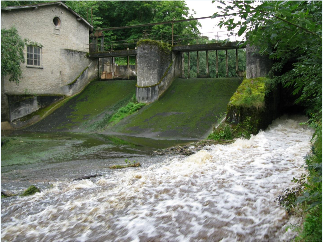
Photo 1. Lower Kunda hydroelectric power station. Note that the upper wooden parts of the dam are missing and all water is (M. Kesler 29.09.2016).
