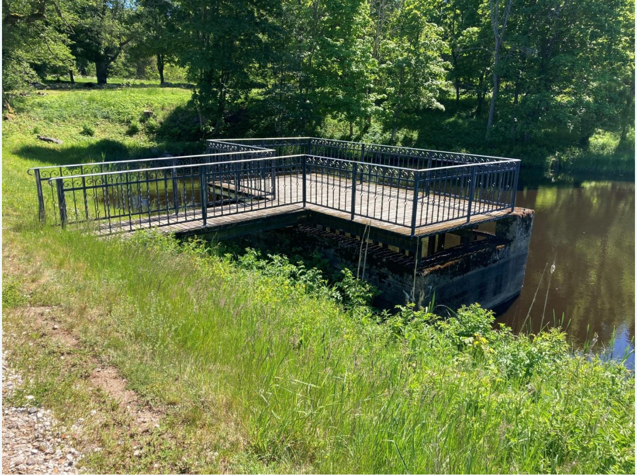
Photo 13. Oandu dam regulator, note that the designed water level is at least one 1 m higher than it is presently maintained.
