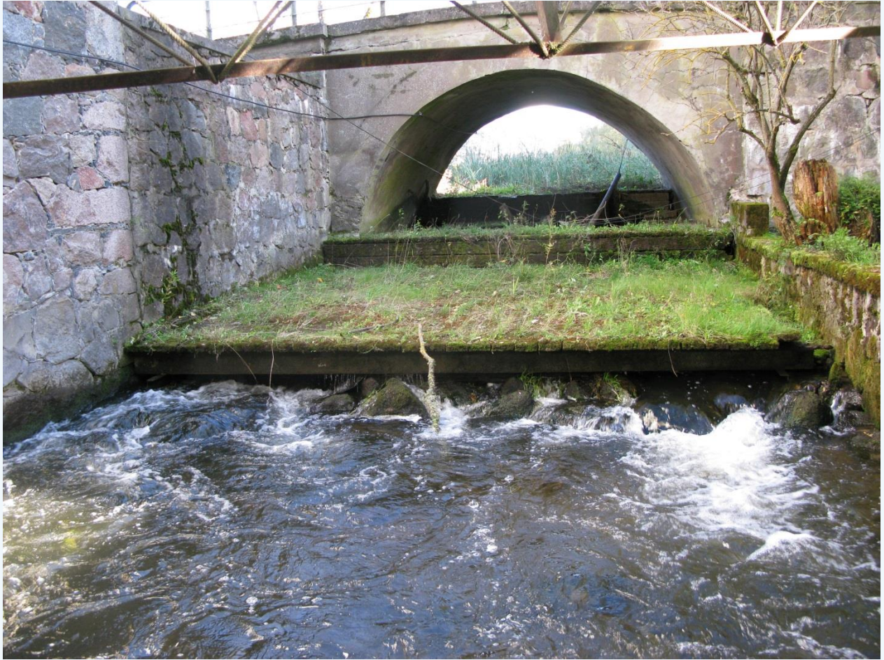
Photo 9. View to Undla dam at r. Loobu. Note that all water flows underneath the upper wooden components of the dam. The dam is located beneath a bridge and that may complicate the full removal of the dam.
