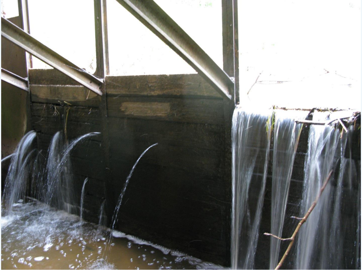
Photo 15. The Kopli dam as a simple metal frame that holds wooden blanks. Removing this structure is very easy.
