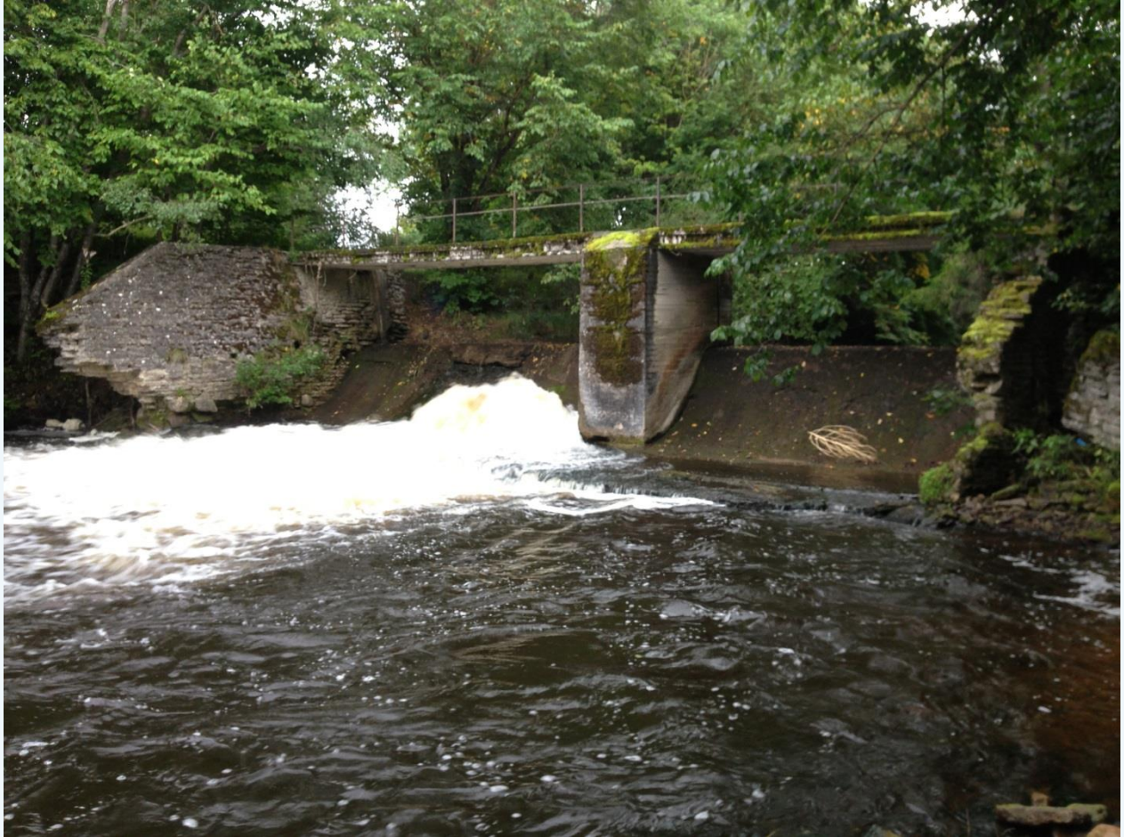
Photo 4. Old Kunda manor mill has no function, is very bad technical condition and is a migration obstacle for fish. The best option is to demolish it (26.07.2019 M. Kesler).
