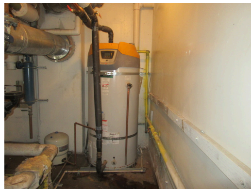
MEP - Building 99 water heater
