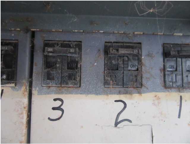
89. MEP - Typical high rise apartment unit electrical main breaker
