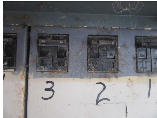
MEP - Typical high rise apartment unit electrical main breaker
