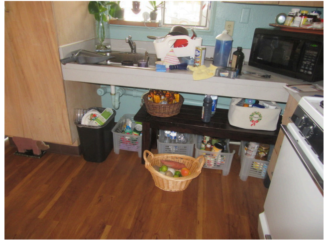
38. Interiors - 79-5 UFAS kitchen sink, need S/A wrap (Critical Repair)
