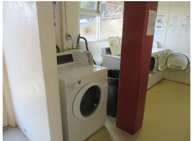
108. Interiors - Building 409 laundry room
