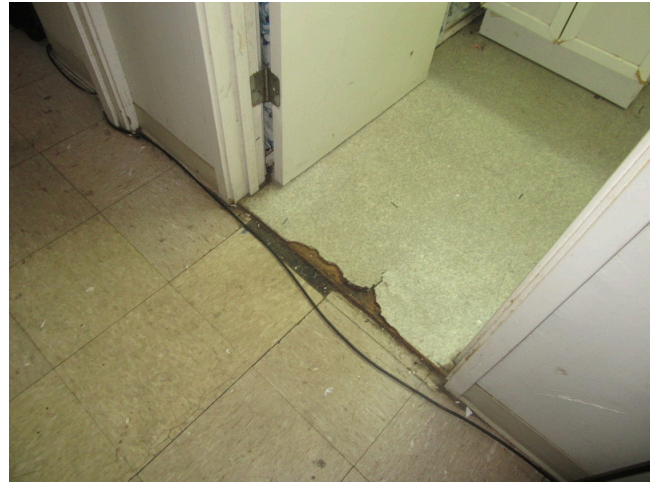
82. Interiors - 387 floor damage
