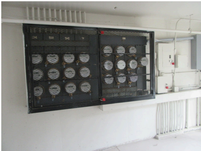
75. MEP - Building 89 electrical meters
