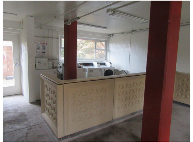
102. Interiors - Building 49 laundry room
