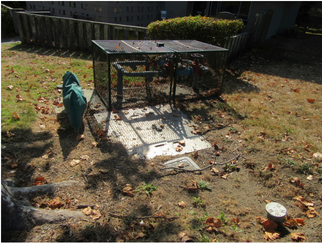
93. MEP - Water backflow preventer near low rise buildings
