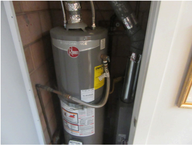
57. MEP - 131 water heater
