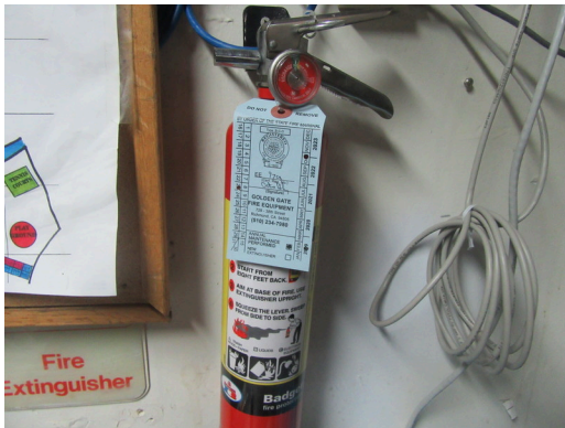
FLS - Fire extinguisher out of date
