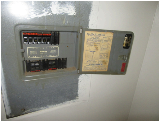
MEP - 25 FPE electrical sub-panel
