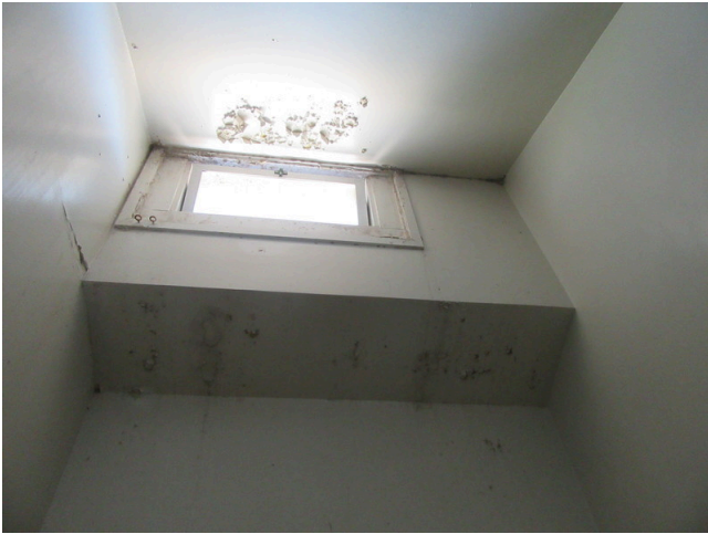
33. Interiors - 72 bathroom high window with water damage (Critical Repair)
