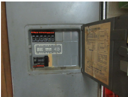
MEP - 50 FPE electrical sub-panel
