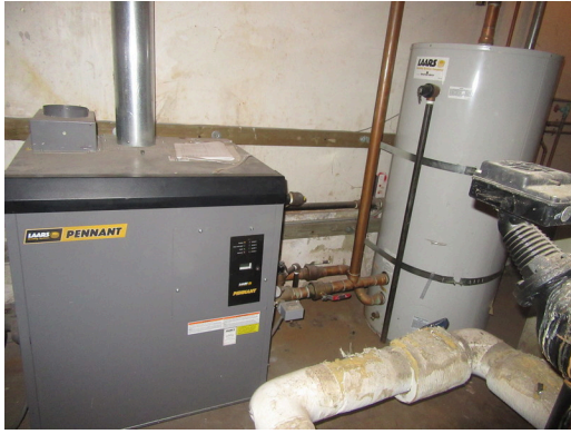
MEP - Building 79 domestic water boiler and storage tank
