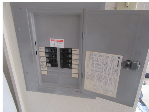
MEP - 419-5 electrical sub-panel
