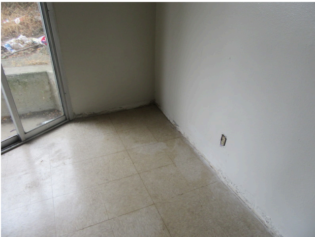
19. Interiors - 49-15 water seepage into the unit (Critical Repair)
