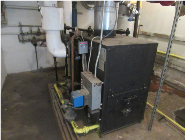
77. MEP - Building 99 boiler
