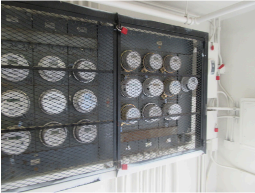
MEP - Building 409 electrical meters
