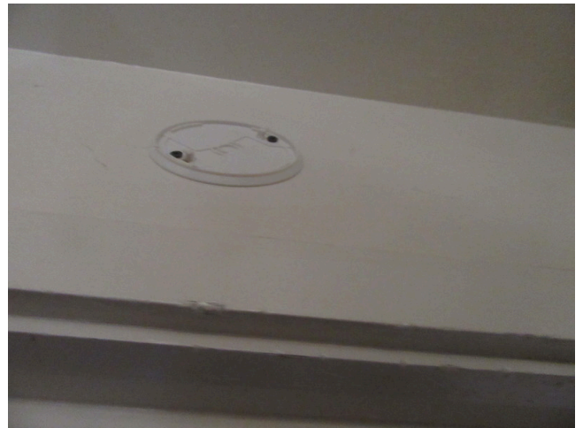
36. FLS - 409-2 missing smoke detector
