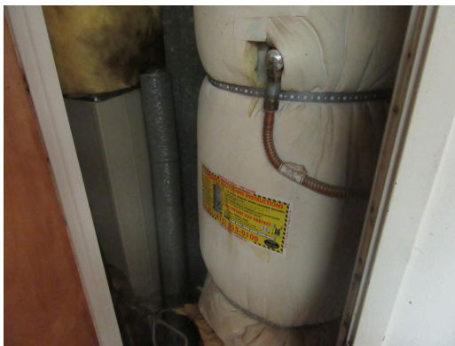
MEP - 255 water heater and furnace
