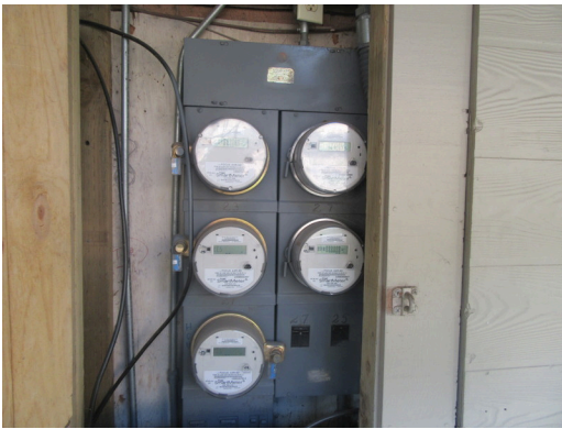
MEP - Lowrise electrical main meters and breakers
