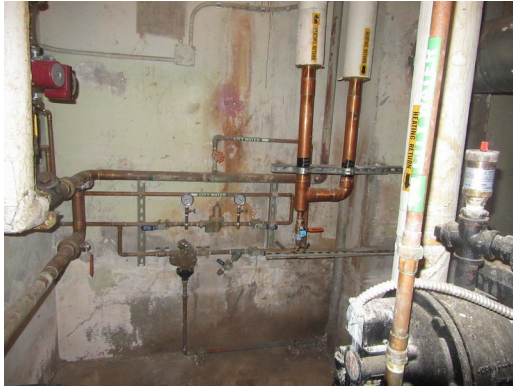
MEP - Water piping
