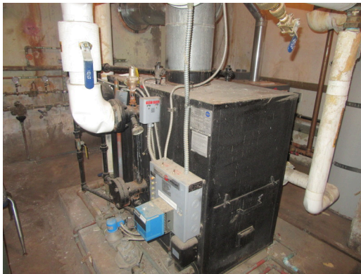
MEP - Building 79 boiler
