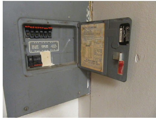
MEP - 37 FPE electrical sub-panel
