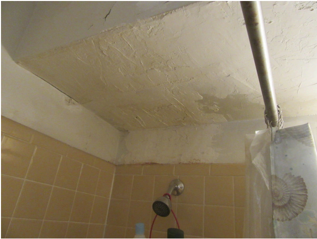
17. Interiors - 49-14 bathroom ceiling damage
