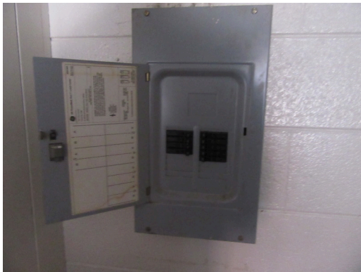
MEP - 129 electrical sub-panel
