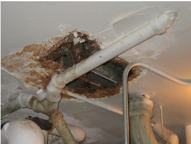
107. Interiors - Building 409 ceiling damage at boiler room
