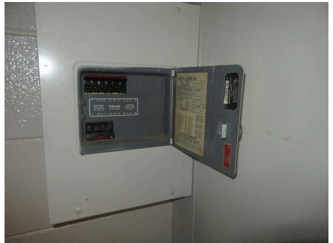
60. MEP - 307 FPE electrical sub-panel
