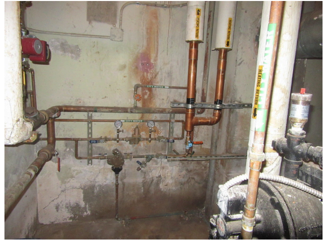
94. MEP - Water piping
