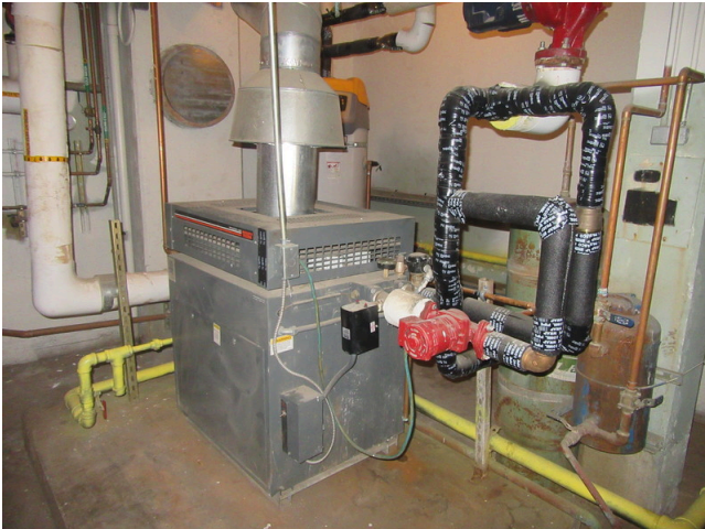
83. MEP - Building 419 boiler
