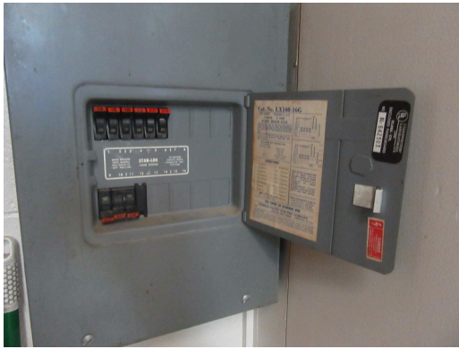
MEP - 72 FPE electrical sub-panel
