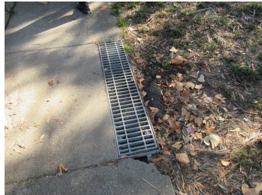
Site - Landscape drain near a walkway
