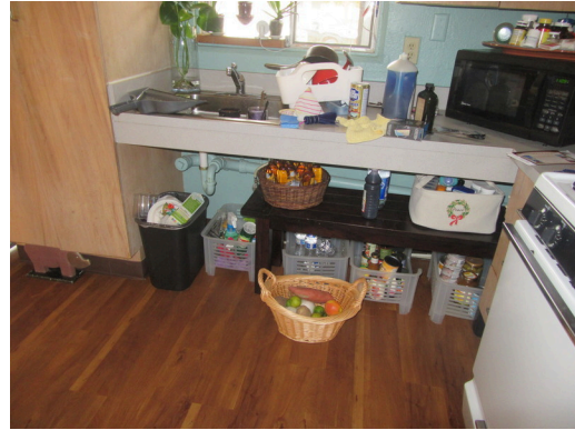
Interiors - 79-5 UFAS kitchen sink, need S/A wrap (Critical Repair)
