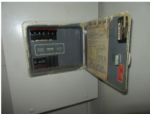
MEP - 387 FPE electrical sub-panel
