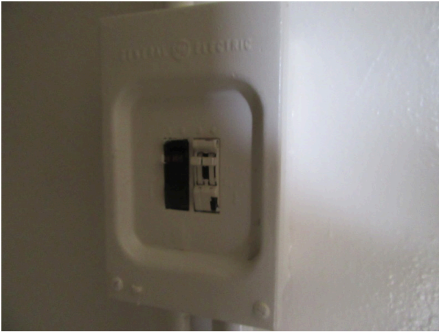
49. MEP - 49-15 electrical sub-panel
