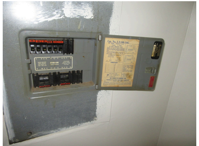
44. MEP - 25 FPE electrical sub-panel
