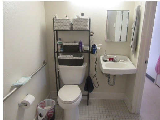
Interiors - 419-5 UFAS bathroom, mirror too high, no s/a wrap
