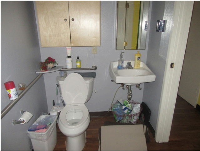
37. Interiors - 79-5 UFAS bathroom, need s/a wrap (Critical Repair)
