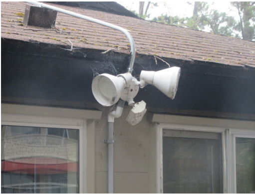
Exterior - Security lighting
