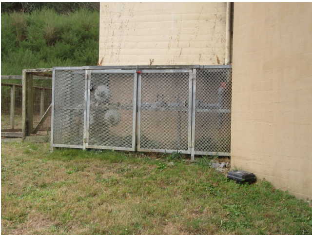
91. MEP - Typical high rise gas meter
