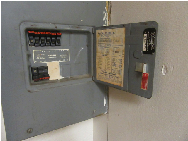
47. MEP - 37 FPE electrical sub-panel
