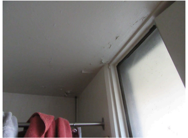
86. Interiors - 409-2 moisture damage at bathroom ceiling
