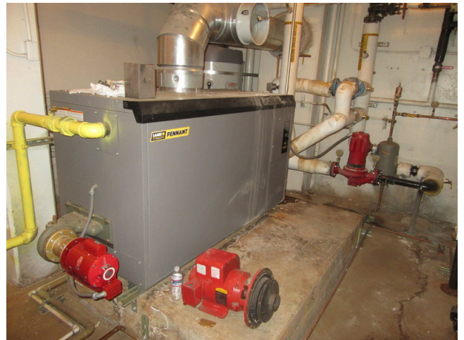
80. MEP - Building 409 boiler
