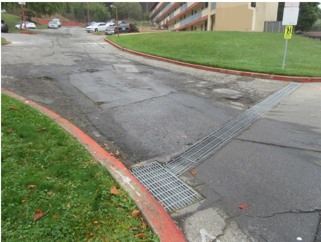
111. Site - Damaged asphalt and trench drain
