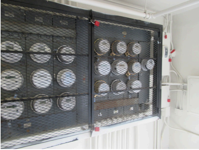
81. MEP - Building 409 electrical meters
