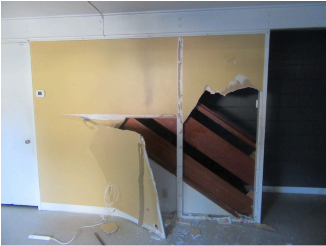
69. Interiors - 211 interior wall at stair infilled by tenant
