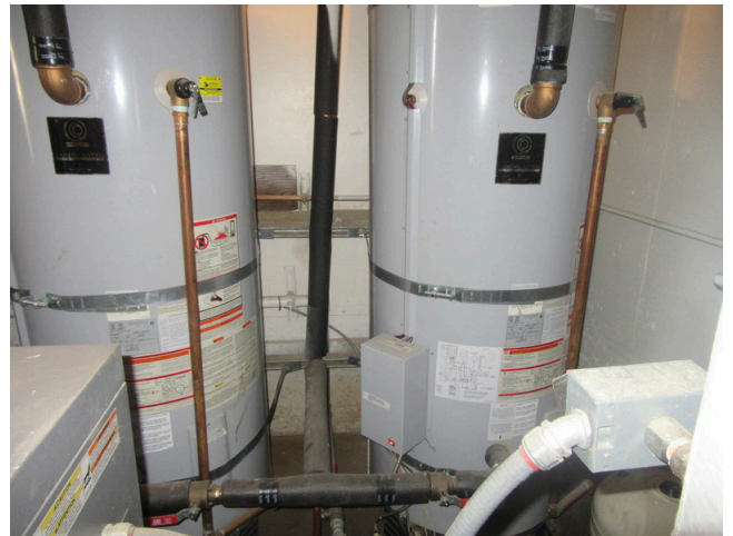
76. MEP - Building 89 water heaters
