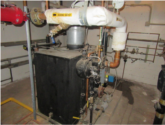
65. MEP - Building 48 boiler
