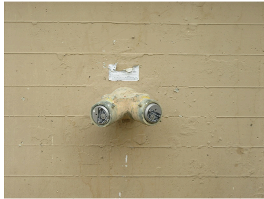
FLS - Fire department connection at highrise
