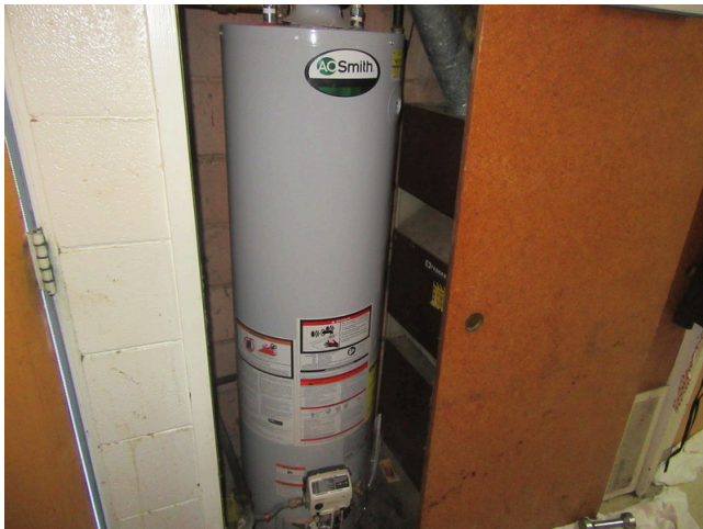
55. MEP - 72 water heater
