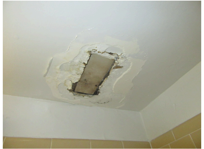
18. Interiors - 49-15 bathroom ceiling damage
