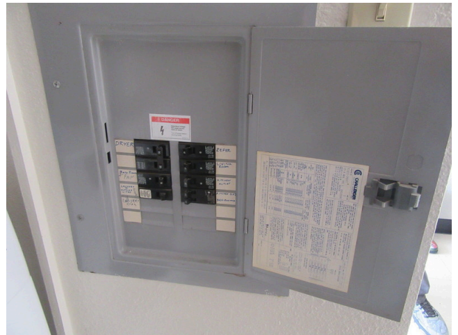
64. MEP - 419-5 electrical sub-panel
