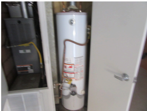
MEP - 25 water heater
