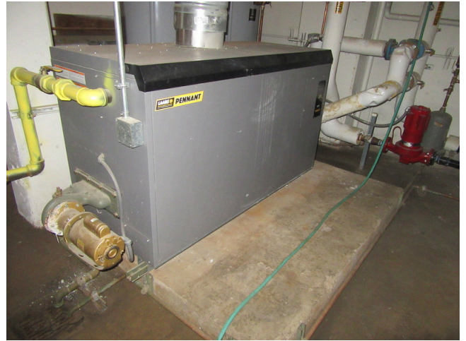
74. MEP - Building 89 boiler
