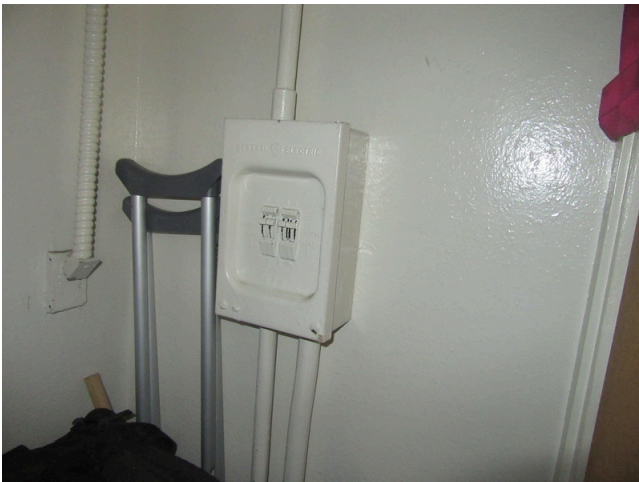
51. MEP - 69-15 electrical sub-panel
