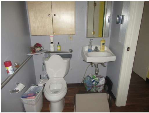
Interiors - 79-5 UFAS bathroom, need s/a wrap (Critical Repair)
