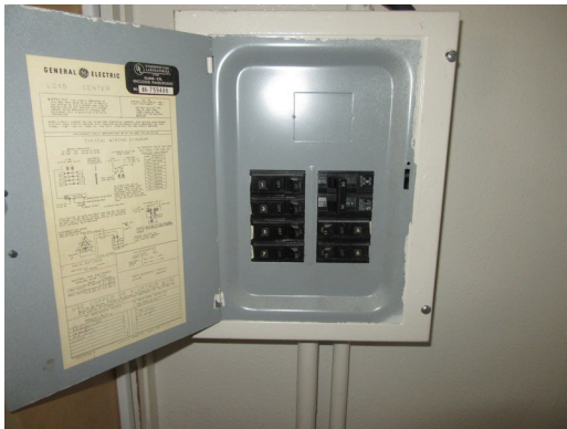
MEP - 49-8 electrical sub-panel
