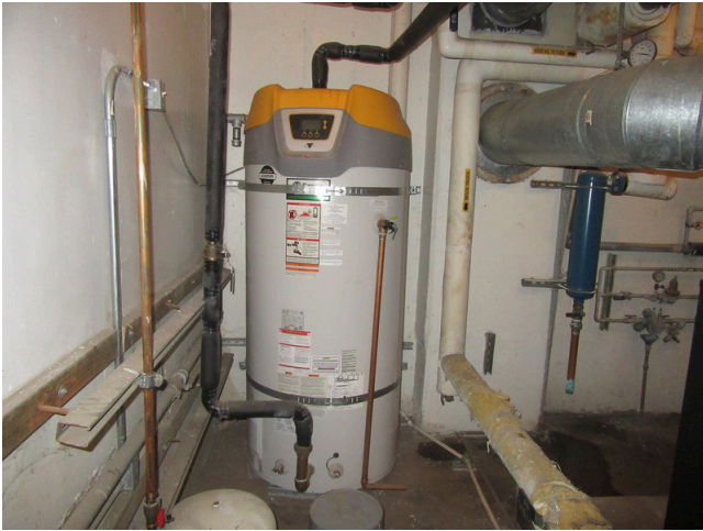
69. MEP - Building 49 water heater
