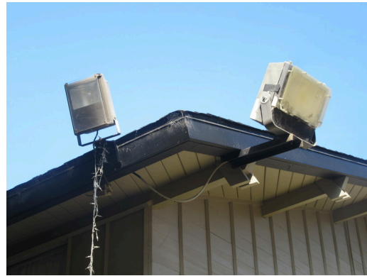
Exterior - Soffit and emergency lighting
