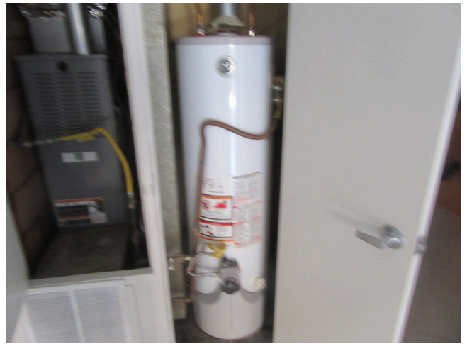
46. MEP - 25 water heater
