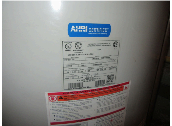
78. MEP - Building 99 water heater tag
