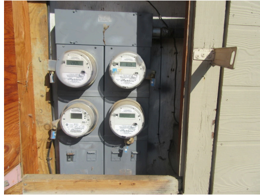
MEP - Lowrise building typical electrical meters
