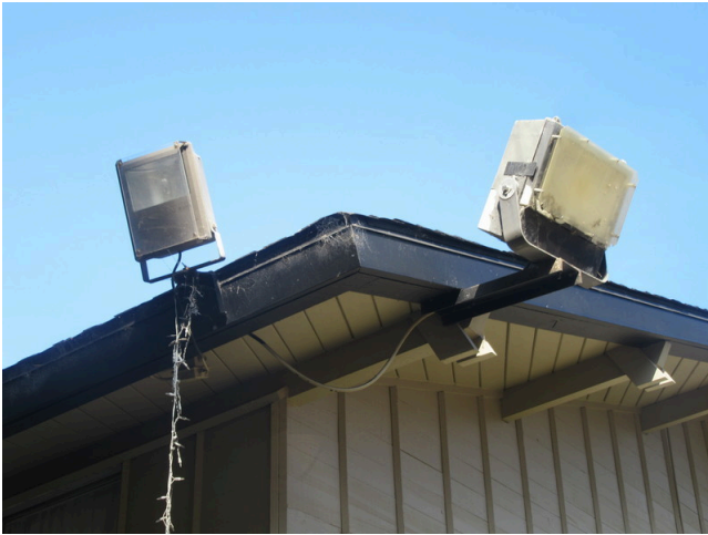
29. Exterior - Soffit and emergency lighting
