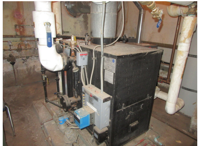
72. MEP - Building 79 boiler
