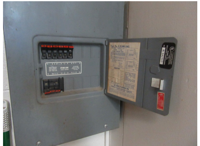
52. MEP - 72 FPE electrical sub-panel
