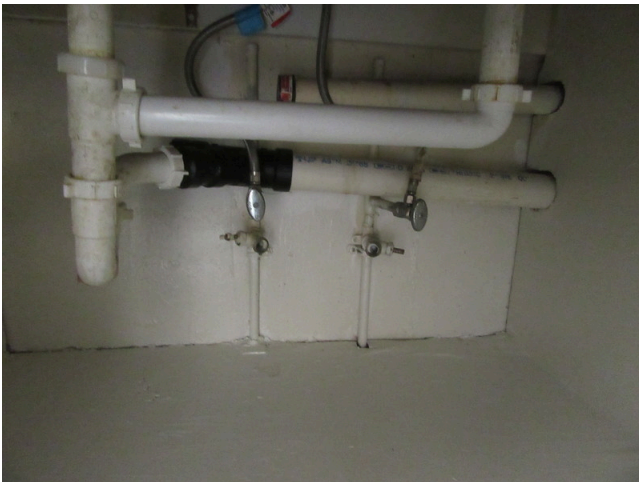
87. MEP - Plumbing piping under the apartment unit kitchen sink
