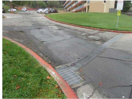
Site - Damaged asphalt and trench drain
