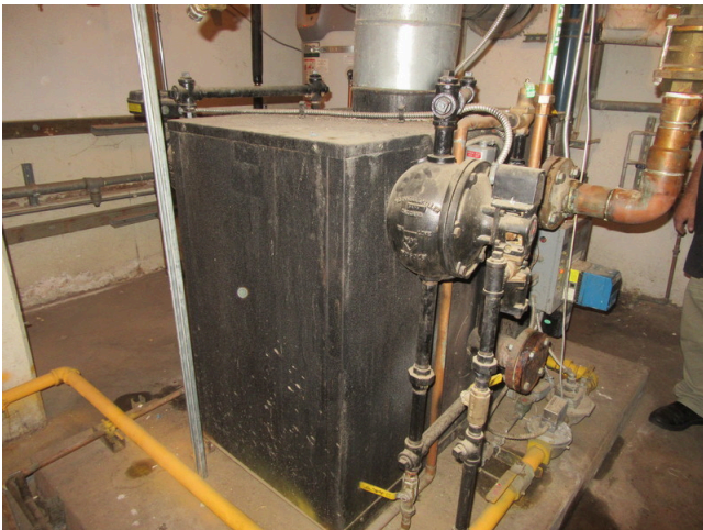
67. MEP - Building 49 boiler
