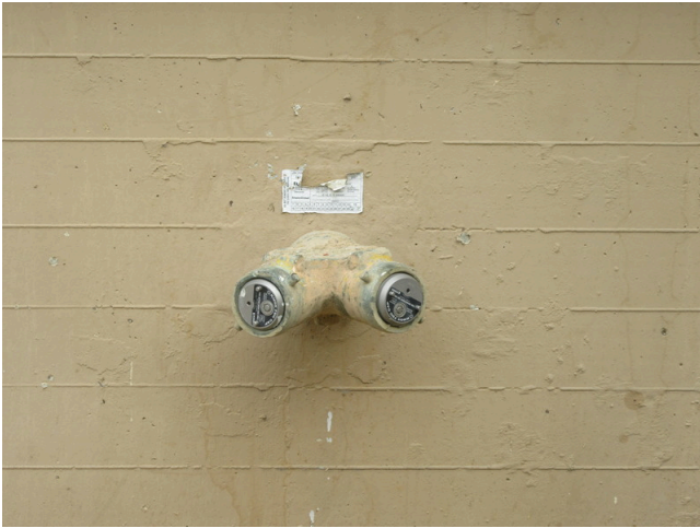
37. FLS - Fire department connection at highrise
