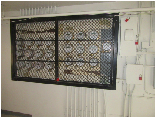
MEP - Typical high rise electrical meters
