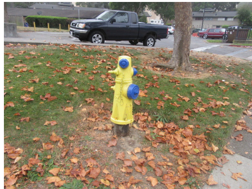
FLS - Fire hydrant
