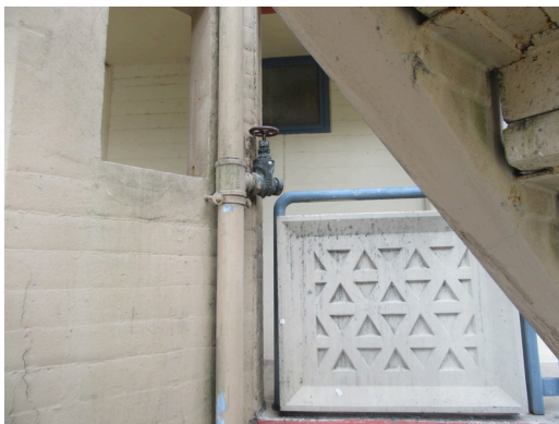
FLS - Highrise standpipe
