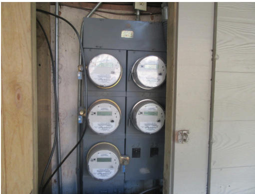
MEP - Lowrise electrical main meters and breakers
