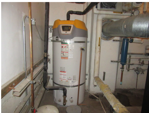
MEP - Building 49 water heater
