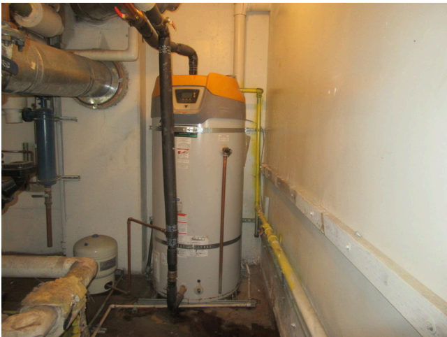
79. MEP - Building 99 water heater
