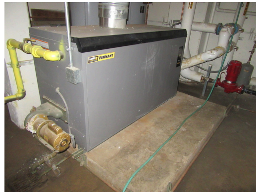
MEP - Building 89 boiler
