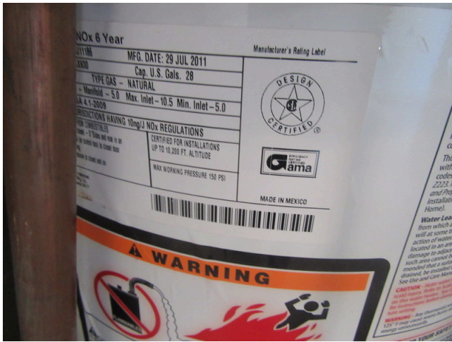
45. MEP - 25 water heater tag
