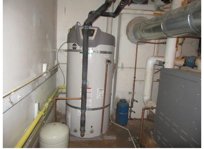
82. MEP - Building 409 water heater
