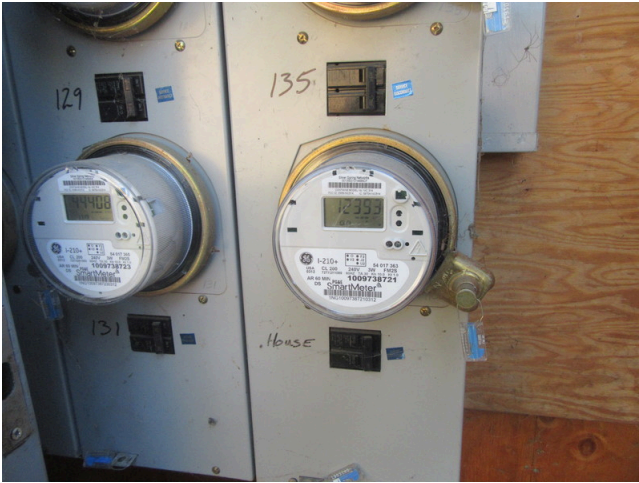
85. MEP - Lowrise building typical electrical meters
