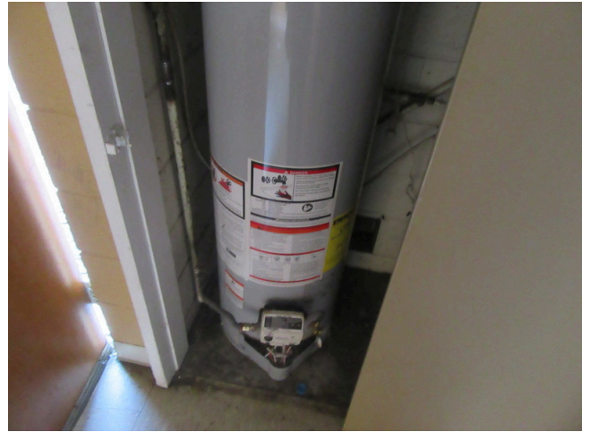
58. MEP - 211 water heater
