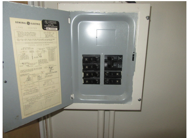
48. MEP - 49-8 electrical sub-panel
