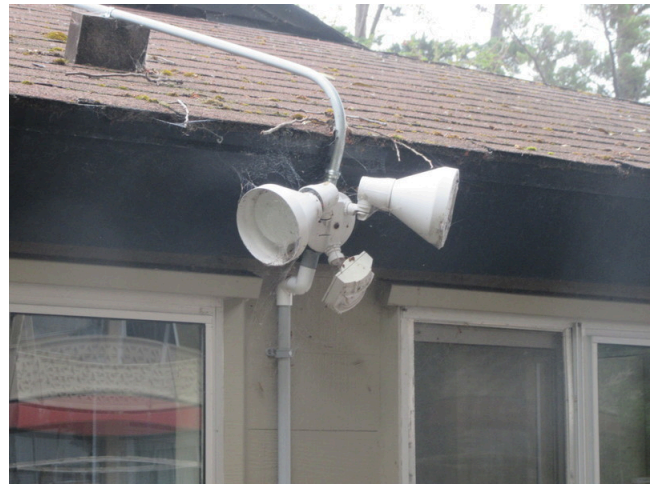
28. Exterior - Security lighting
