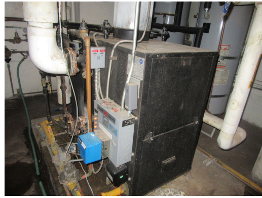
MEP - Building 59 boiler
