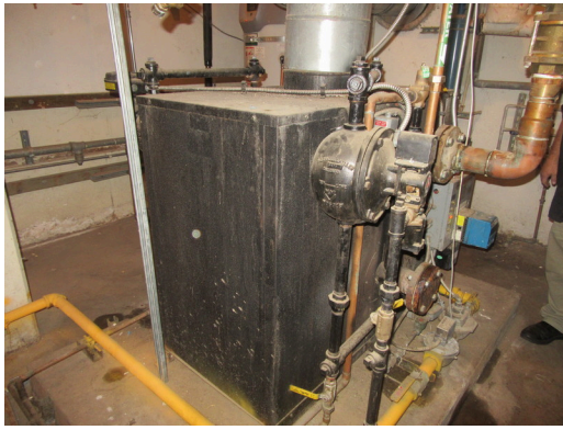
MEP - Building 49 boiler
