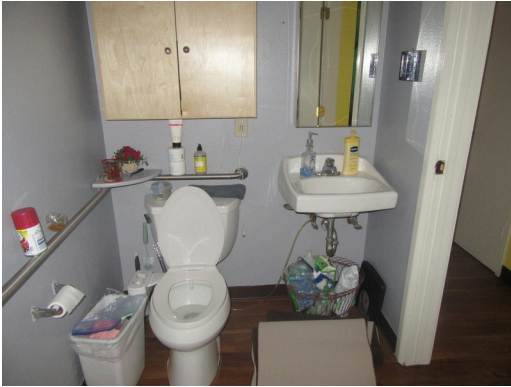
Interiors - 79-5 UFAS bathroom, need s/a wrap (Critical Repair)
