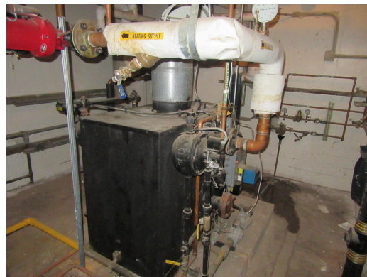
MEP - Building 48 boiler
