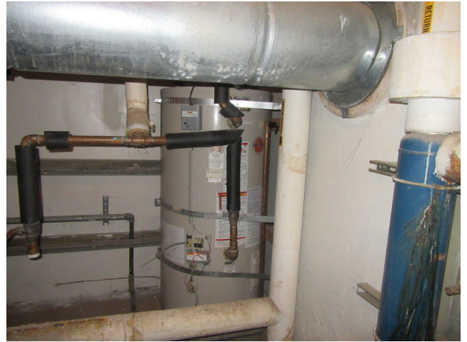
66. MEP - Building 48 water heater
