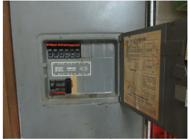
50. MEP - 50 FPE electrical sub-panel
