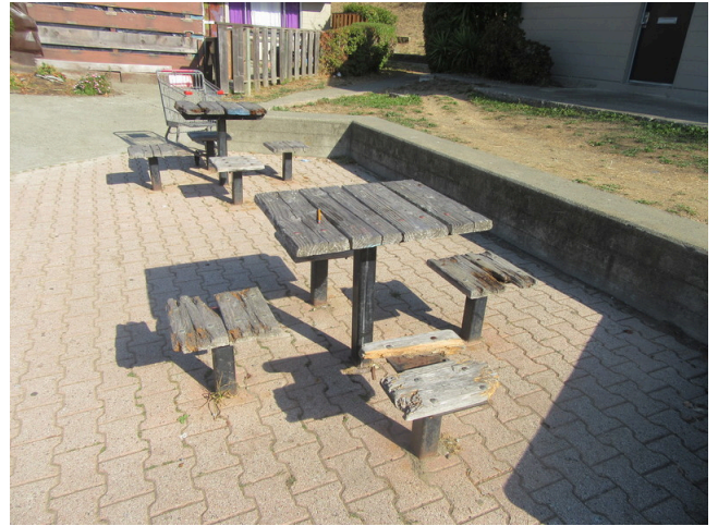
110. Site - Courtyard table and seats heavily weathered
