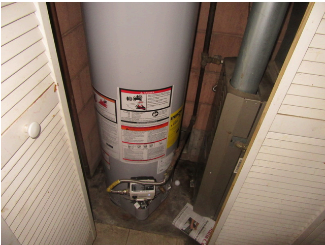
63. MEP - 387 water heater
