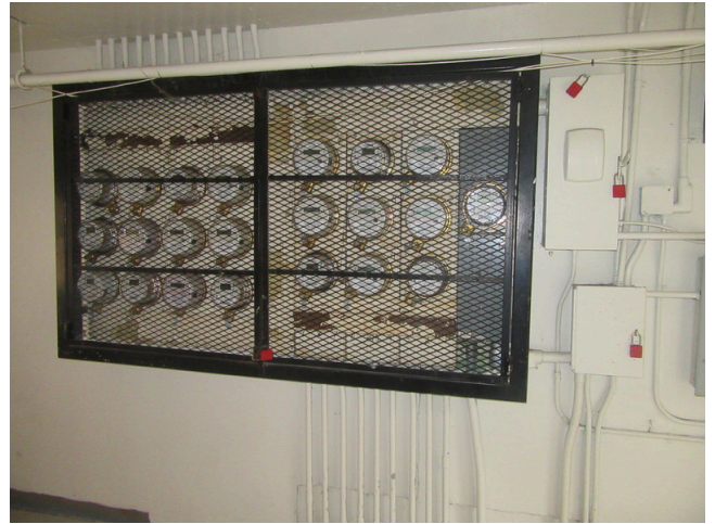
90. MEP - Typical high rise electrical meters
