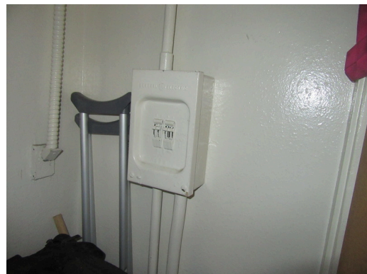
MEP - 69-15 electrical sub-panel
