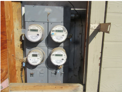
MEP - Lowrise building typical electrical meters
