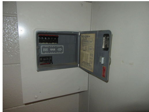
MEP - 307 FPE electrical sub-panel
