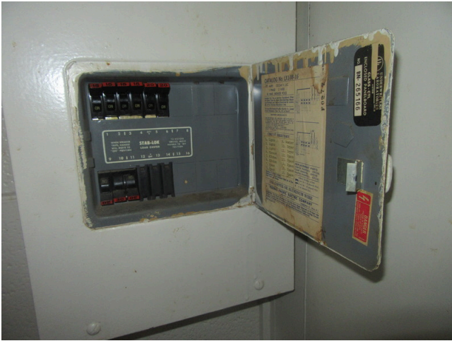
61. MEP - 387 FPE electrical sub-panel
