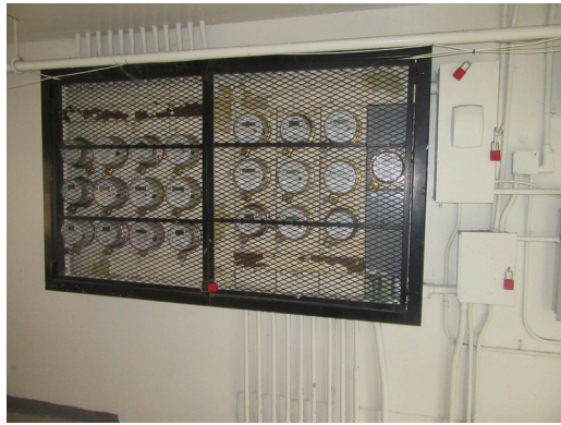
MEP - Typical high rise electrical meters
