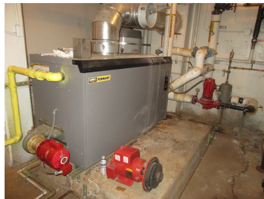
MEP - Building 409 boiler
