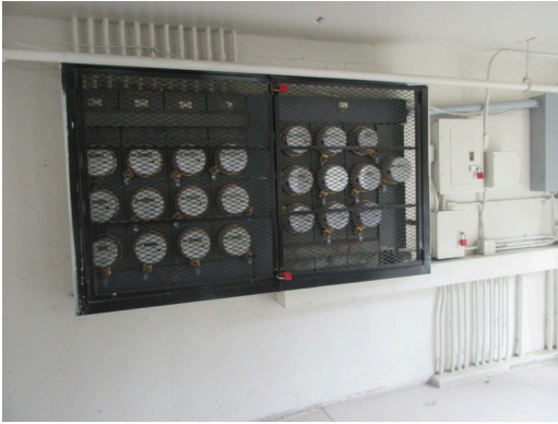
MEP - Building 89 electrical meters
