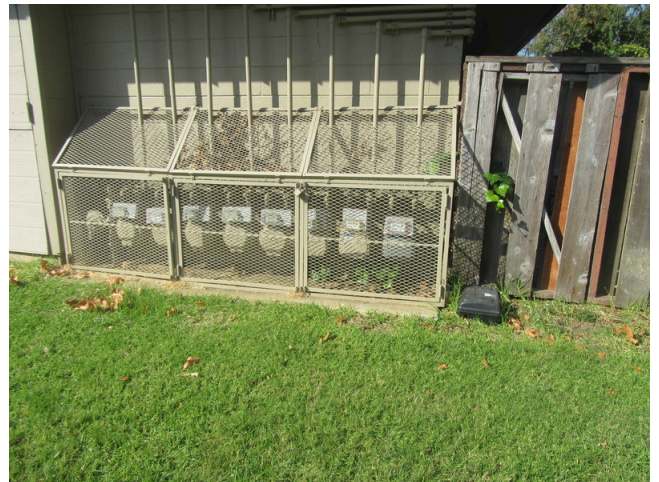
92. MEP - Typical low rise building gas meters
