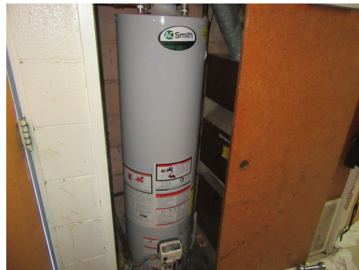
MEP - 72 water heater
