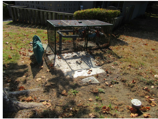
MEP - Water backflow preventer near low rise buildings
