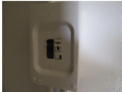
MEP - 49-15 electrical sub-panel
