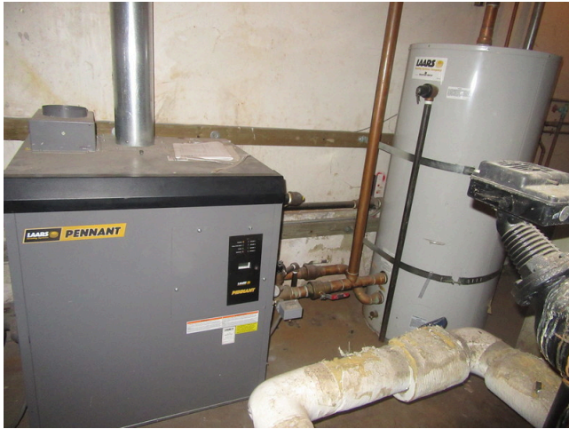
73. MEP - Building 79 domestic water boiler and storage tank
