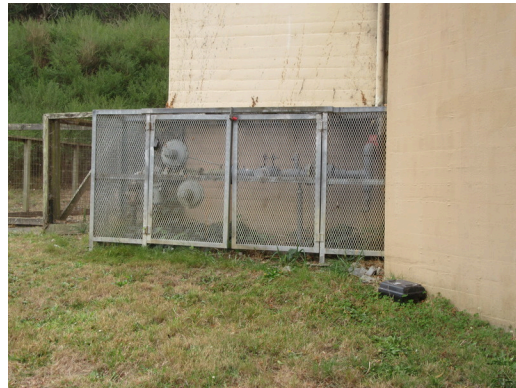
MEP - Typical high rise gas meter
