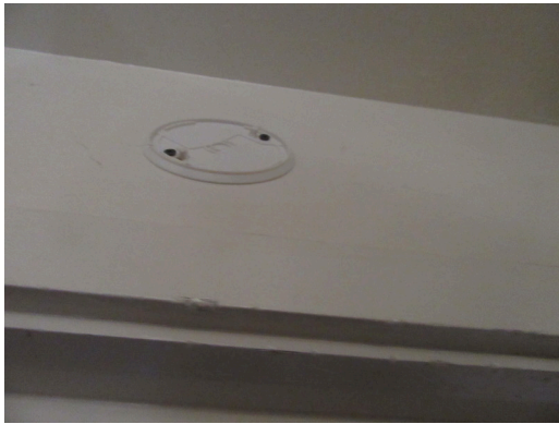
FLS - 409-2 missing smoke detector
