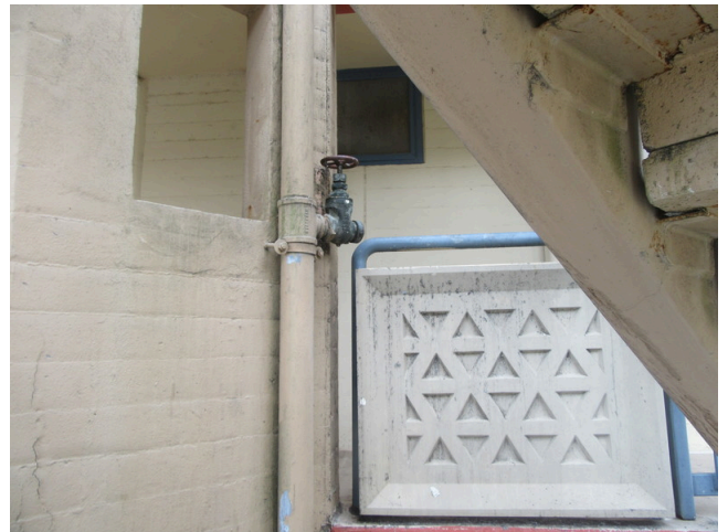
40. FLS - Highrise standpipe
