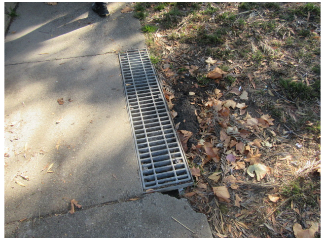
116. Site - Landscape drain near a walkway
