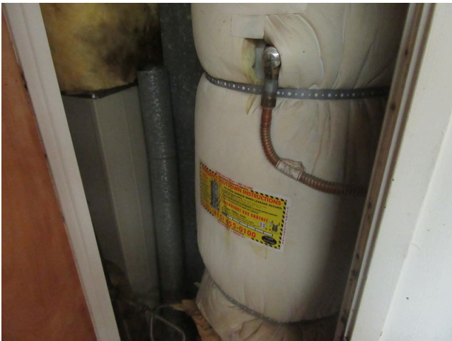
59. MEP - 255 water heater and furnace
