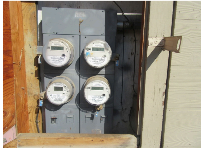
84. MEP - Lowrise building typical electrical meters
