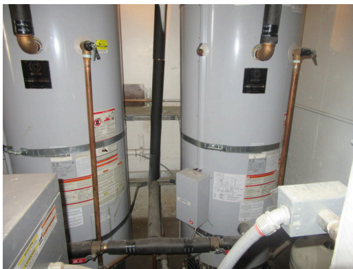
MEP - Building 89 water heaters
