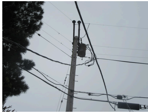
MEP - Pole mounted electrical transformer
