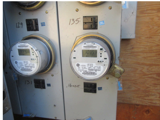
MEP - Lowrise building typical electrical meters
