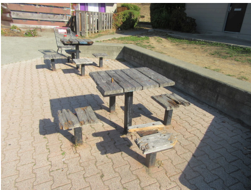
Site - Courtyard table and seats heavily weathered
