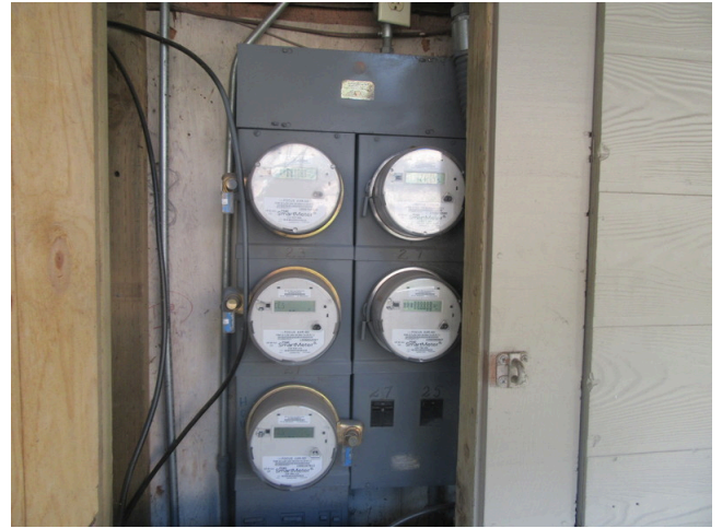
86. MEP - Lowrise electrical main meters and breakers
