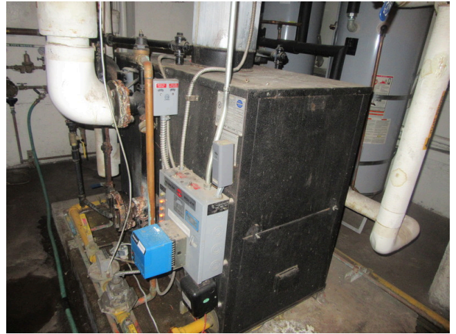
70. MEP - Building 59 boiler
