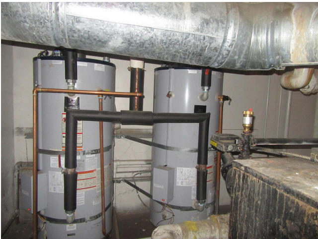
71. MEP - Building 59 water heaters
