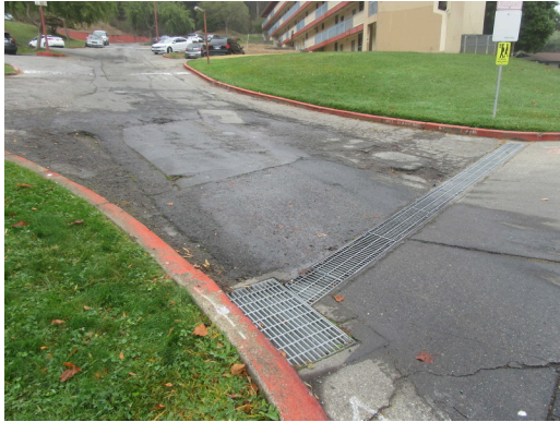
Site - Damaged asphalt and trench drain
