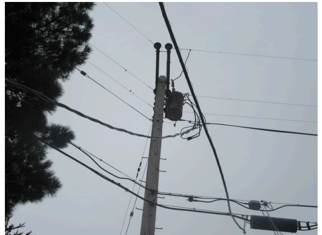
88. MEP - Pole mounted electrical transformer
