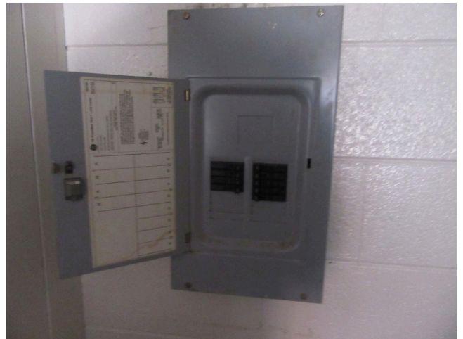
56. MEP - 129 electrical sub-panel
