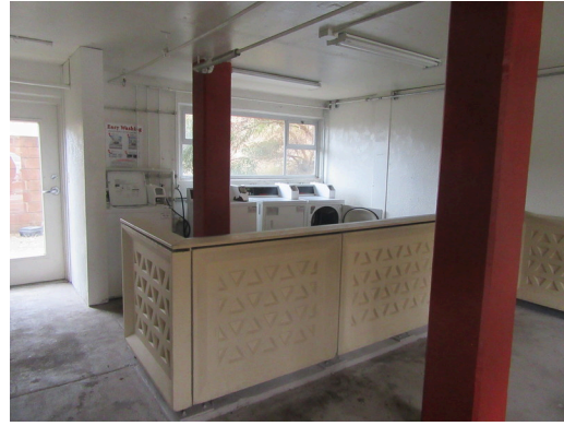
Interiors - Building 49 laundry room
