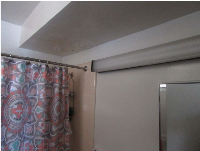
95. Interiors - 419-9 bathroom soffit damage
