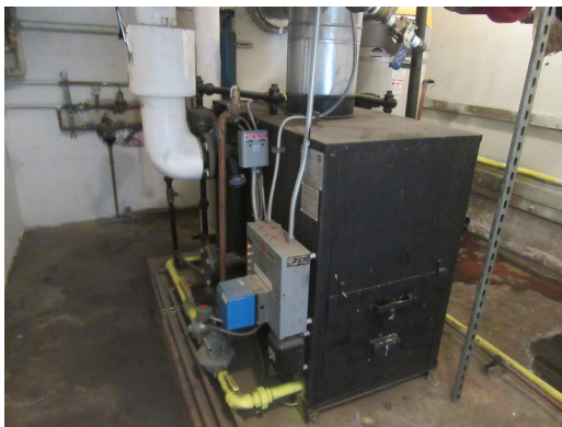
MEP - Building 99 boiler
