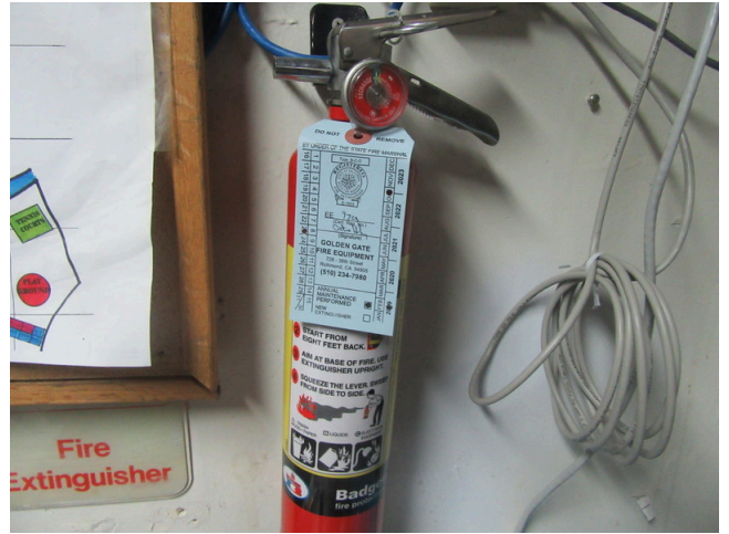
38. FLS - Fire extinguisher out of date
