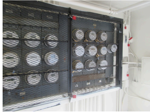
MEP - Building 409 electrical meters
