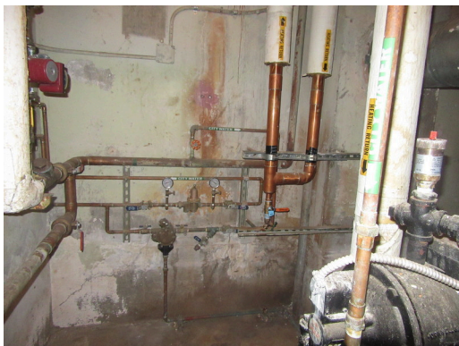
MEP - Water piping
