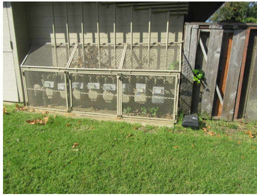
MEP - Typical low rise building gas meters
