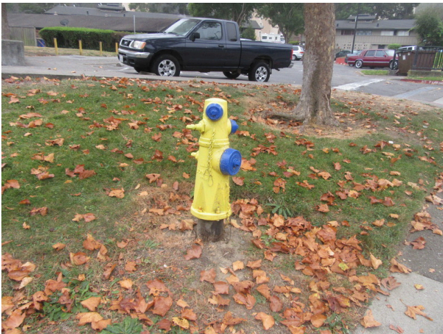
39. FLS - Fire hydrant
