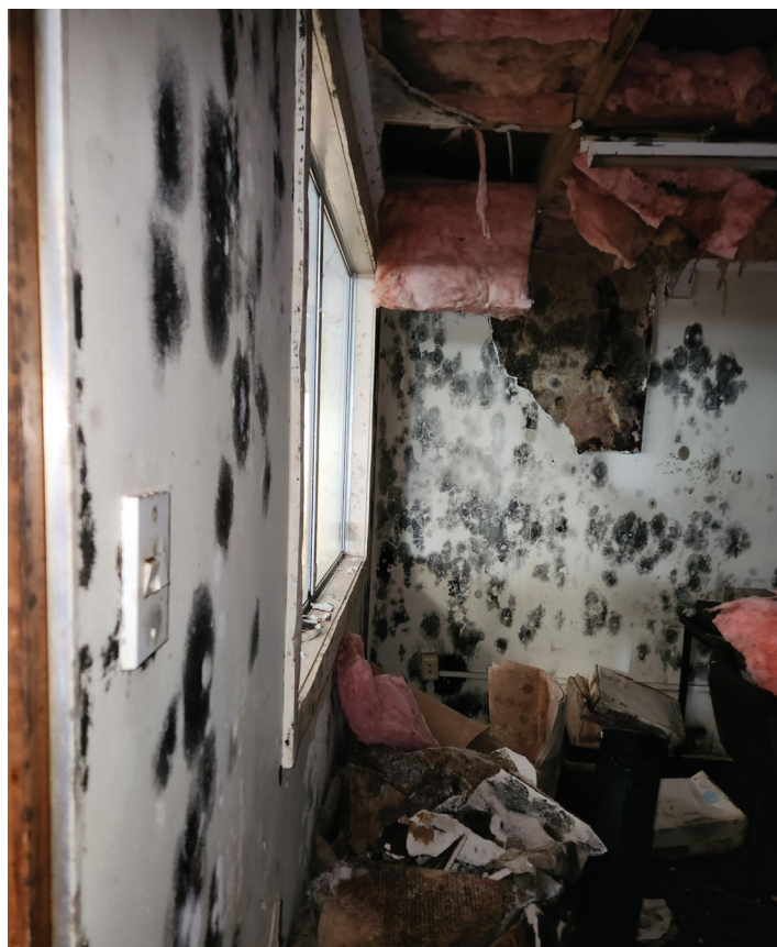
A very mouldy room with toxic mould
