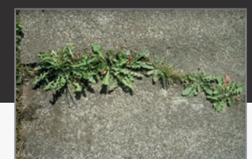
Weeds on pavement
