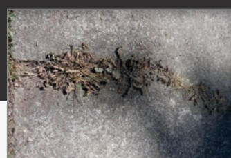
Weeds on pavement 2 - 5 days after treatment
