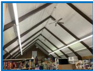
Convert lighting to LED.
