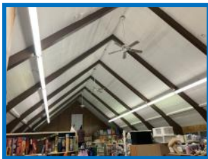
Convert lighting to LED.
