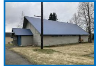
Replace all windows.
