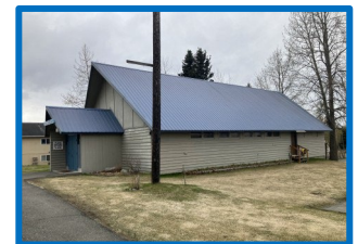
Replace all windows.
