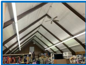
Convert lighting to LED.
