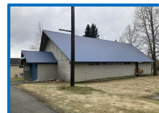
Replace all windows.
