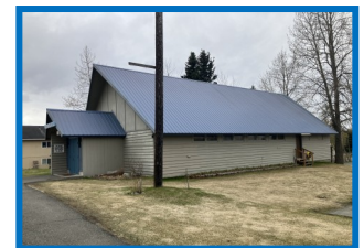
Replace all windows.
