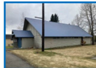
Replace all windows.
