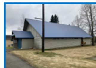
Replace all windows.
