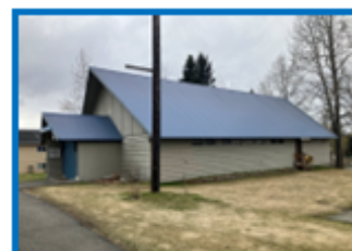
Replace all windows.
