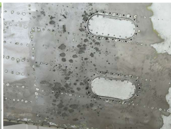
Closeup of Corrosion (dark pits)
