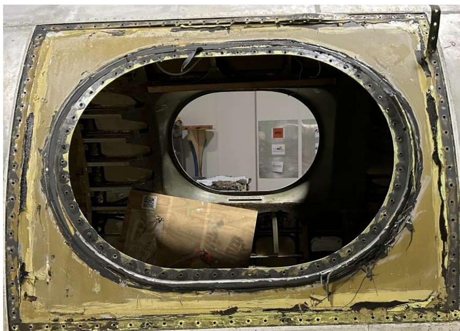
Left cabin window removed – Open emergency hatch in background
