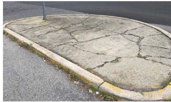
FIGURE 12: NON-COMPLIANT REFUGE ISLAND (DUE TO LARGE CRACKS AND LACK OF CURB RAMPS)
