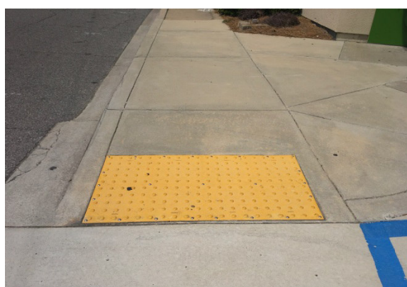
FIGURE 3: COMPLIANT CURB RAMP
