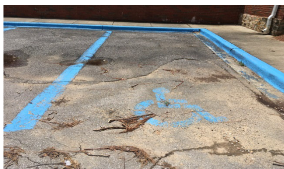
FIGURE 8: NON-COMPLIANT ACCESSIBLE PARKING AREA (DUE TO LACK OF BOTH SIGNAGE AND ACCESS AISLE AND PAVEMENT DETERIORATION)
