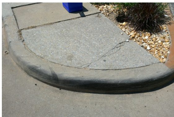
FIGURE 13, TO LEFT: NON-COMPLIANT OTHER FEATURE (DUE TO LACK OF A RAMP)
