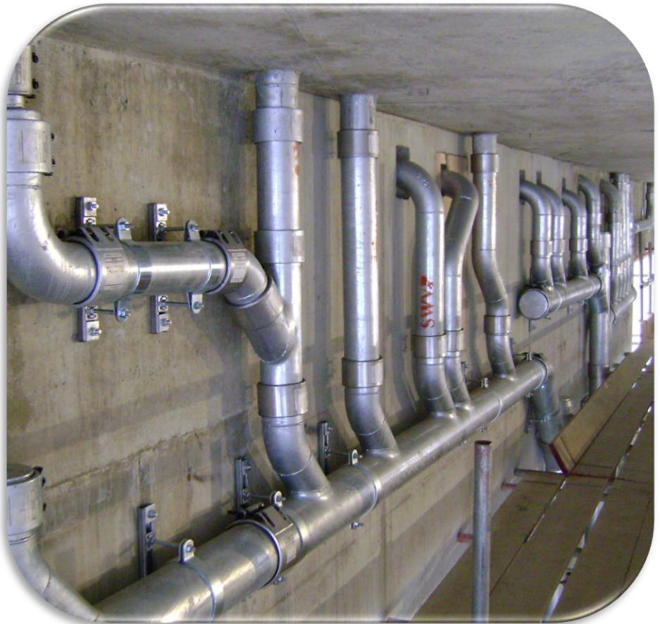
Picture shows pipe work installed at the One Hyde Park. Apartments
