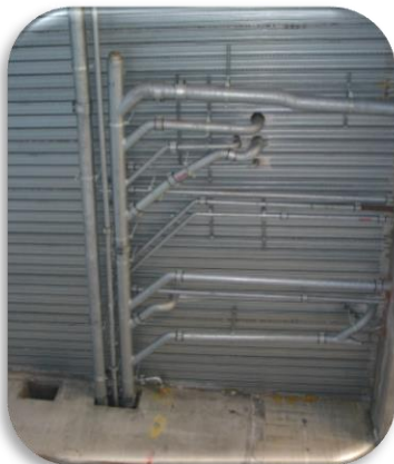
Pipework under slab on apartment contract in Battersea
