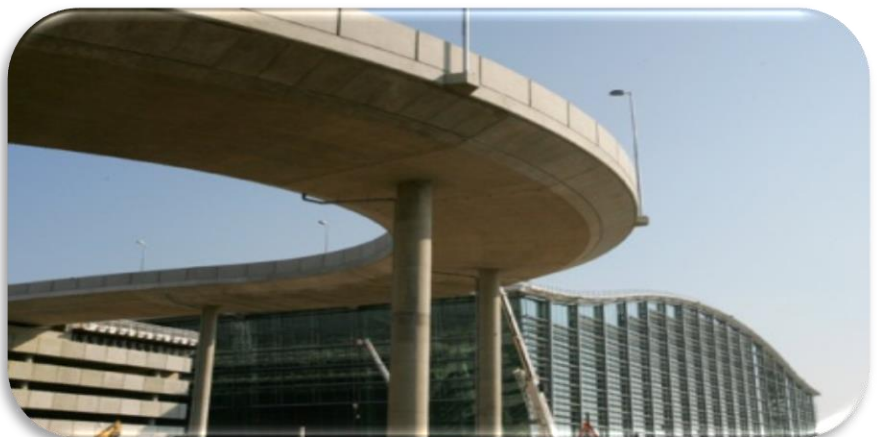
Rainwater pipes running up the support column at T5 Heathrow
