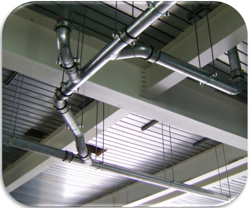
Picture shows pipe work installed at the Heathrow T5c.
