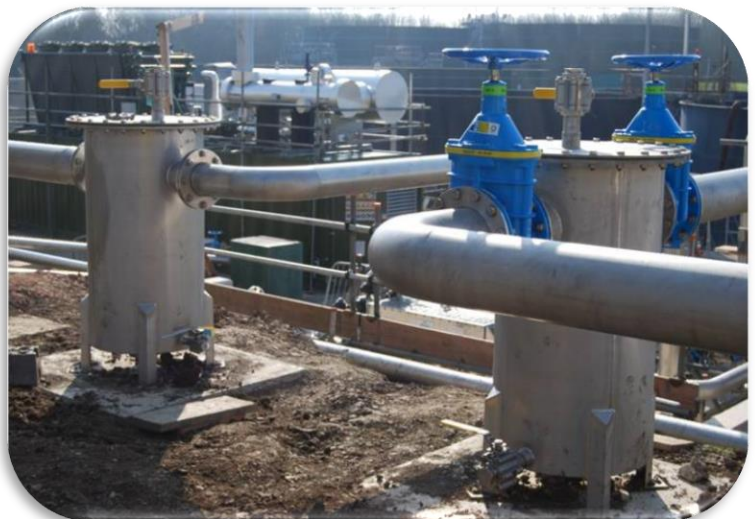
Stainless steel tanks and flanged pipework
