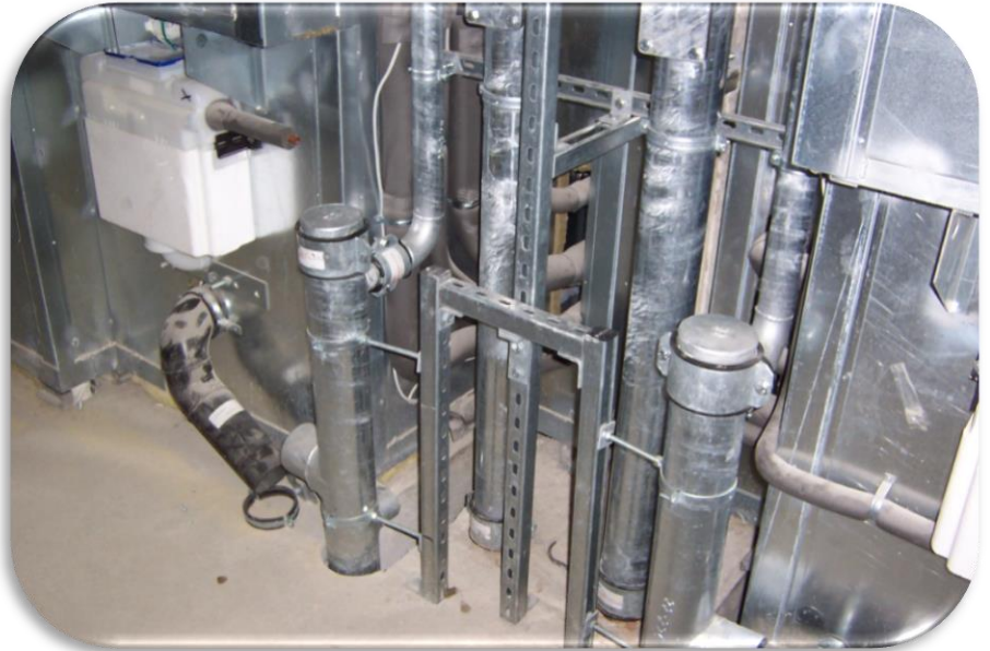
Galvanised pipework connecting onto bathroom pods
