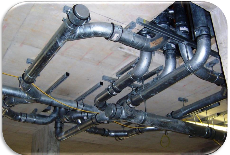
Drainage pipework serving vertical risers in a confined duct space
