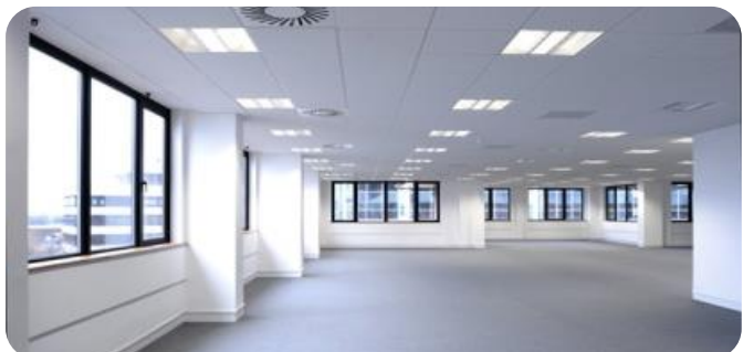
False ceiling containing galvanised steel drainage pipework
