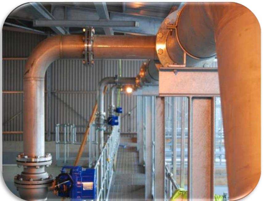
Pipe supports for stainless steel pipes
