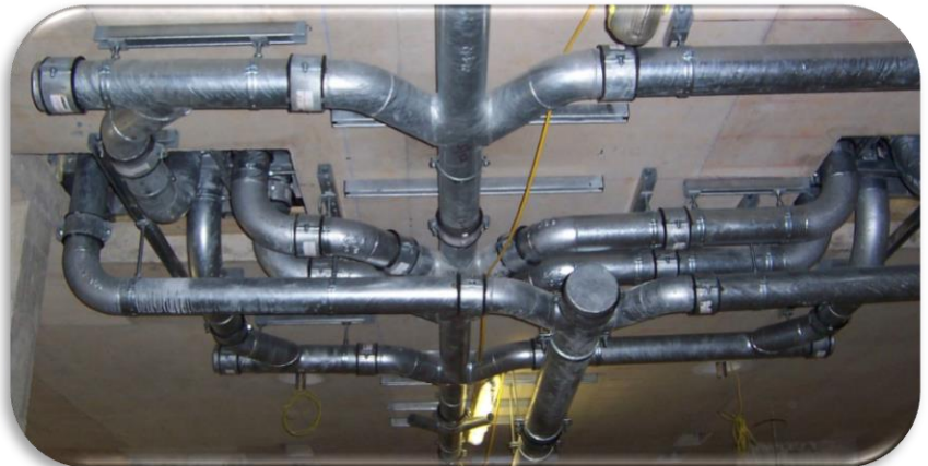
Galvanised pipework serving service ducts each side of a hotel corridor
