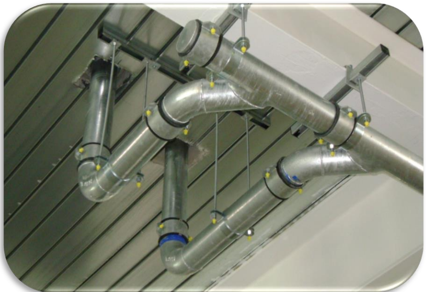
Pipe work installed over sensitive area all rodding from floor above.
