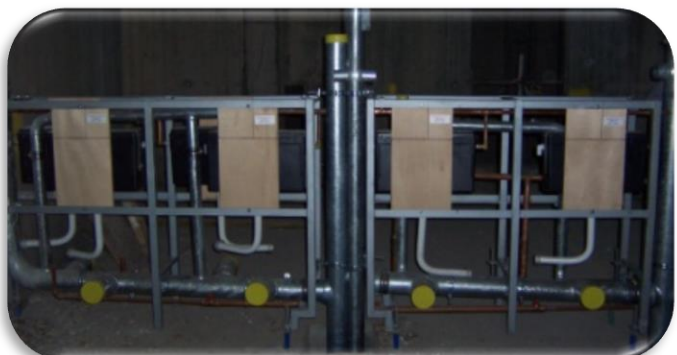
Galvanised steel manifold in frame with cisterns and service pipe
