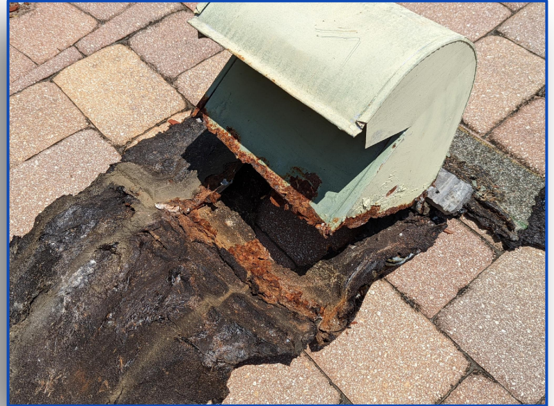
GRV roof vent failure at roof line due to chemical cleaning.
