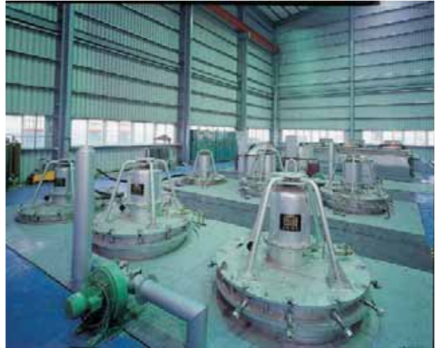
Quench & Tempered Facility
