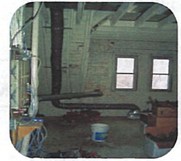
Attic with buckets catching rain drops!
