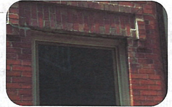
Deteriorating window lentil
