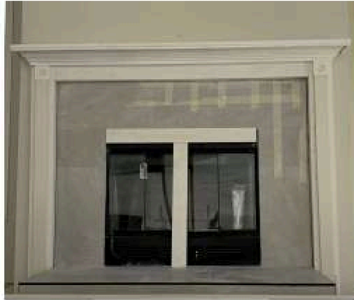
WOOD BURNING FIREPLACE WITH HEARTH
