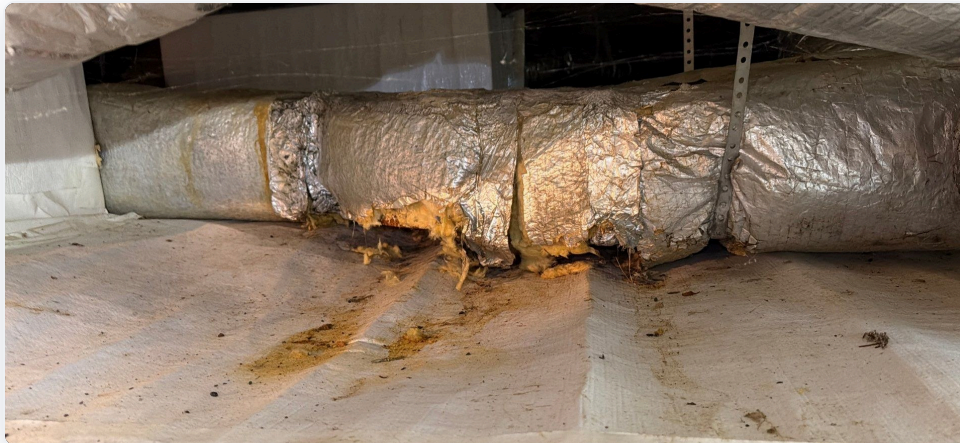
Figure 4. Saturated duct insulation that has sagged to the crawl space floor, with water staining on the ground cover. Coastal Virginia.
