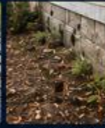
Severe erosion or washout
