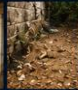
Erosion starting near foundation
