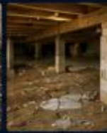
Damp or musty crawlspace
