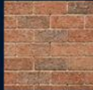
Hairline brick crack
