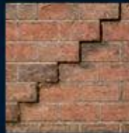
Large stair-step brick cracking
