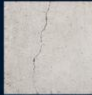
Hairline shrinkage crack
