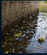
Standing water near foundation
