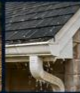
Gutters overflowing during storms
