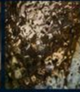
Chronic moisture and mold
