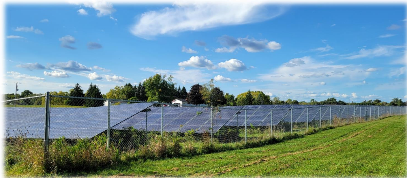
Onsted Schools Solar Project
