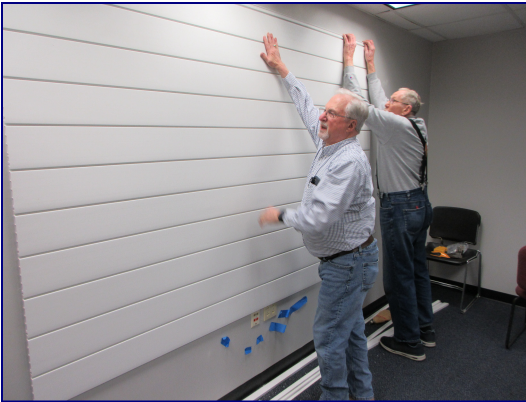
At left, Steve Cohn and Al Firnrohr are shown during a recent work party preparing one of the walls in the room adjacent to the “P-3 Room” with slat-boards so we can hang up more framed photos and other artifacts in there. This room has a large built-in bookcase and may end up as a library and reading room for researchers.
