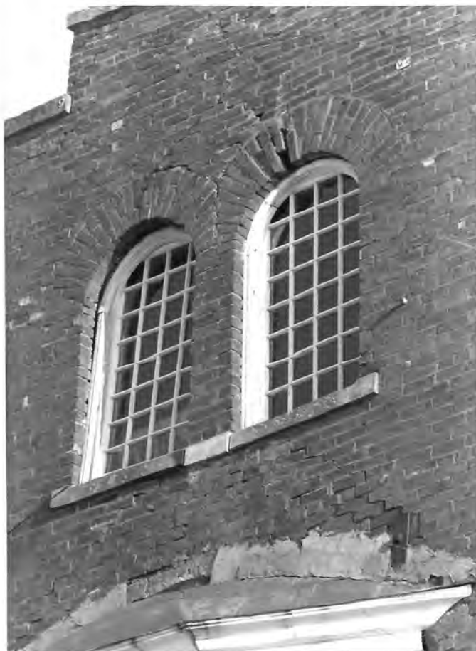
Fig. 28. Evidence of cracks extending to the third floor above the bay window on the west facade.
