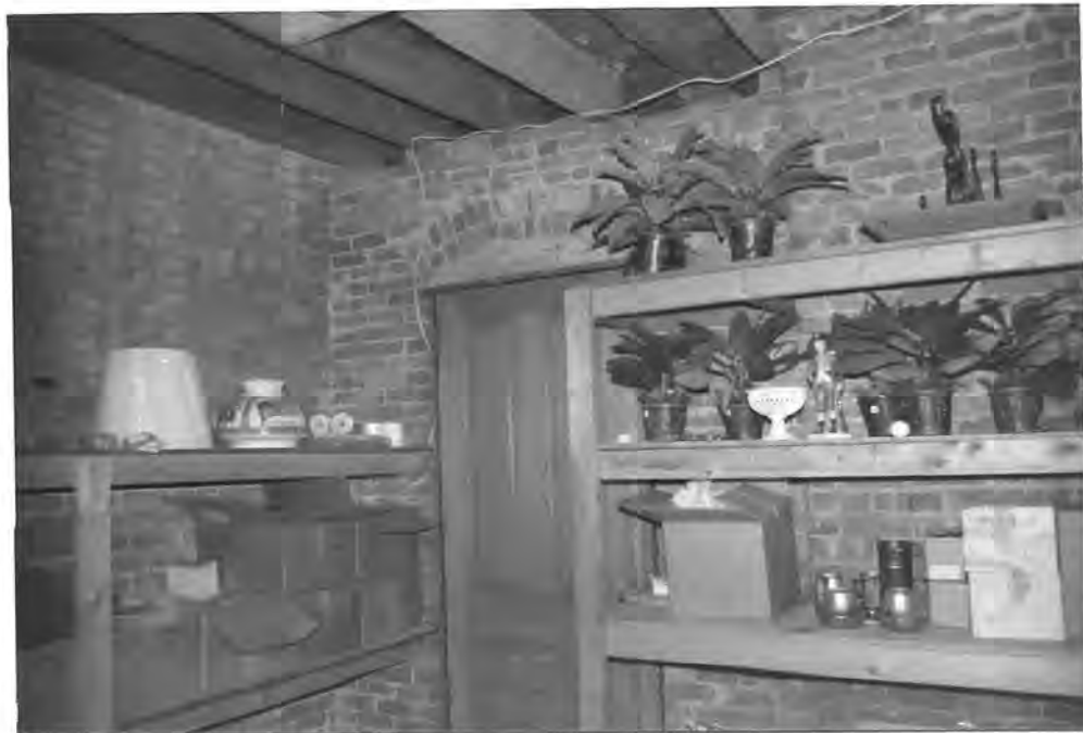
Fig. 47. Room 201. Exposed brick on west wall which could be kept for aesthetic reasons.
