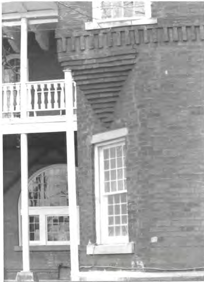
Fig. 27. Crack extending from ground level to cantilevered corner.
