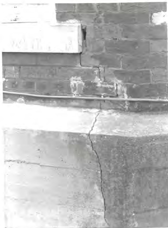
Fig. 29. Exterior reinforcement walls have cracked with the shifting of the house.
