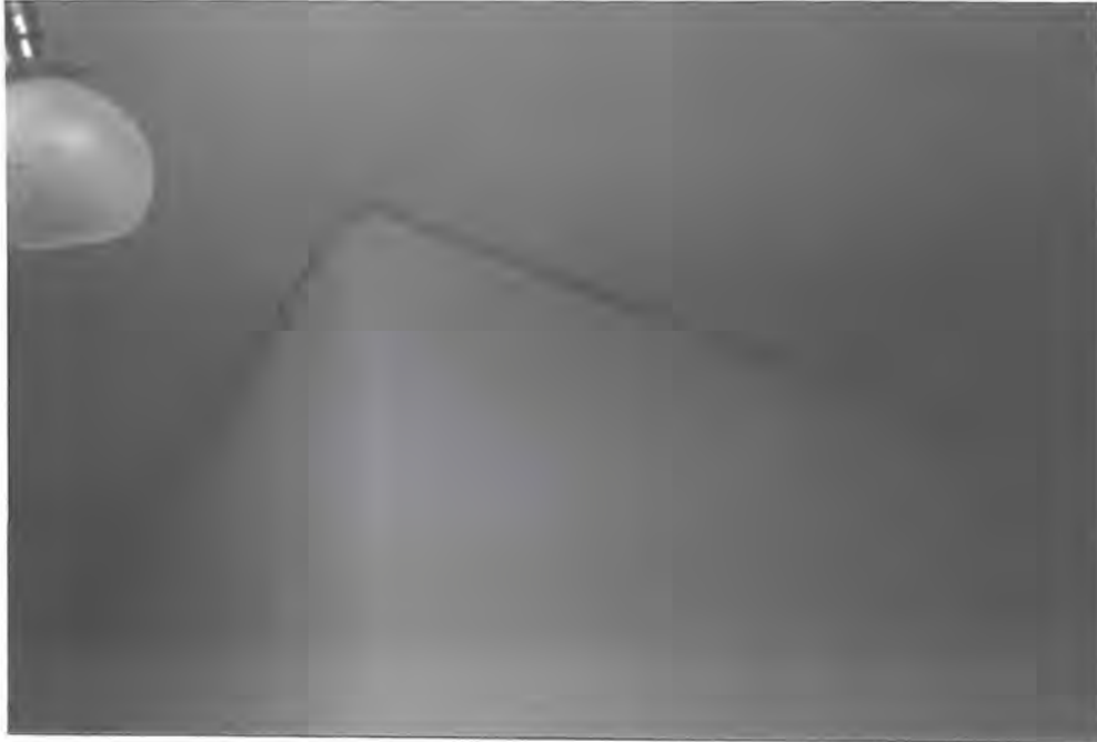
Fig. 42. Ceiling and wall separation in room 204.
