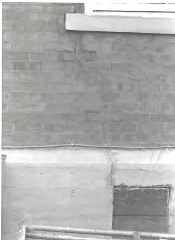
Fig. 26. Structural cracks begin at ground level.
