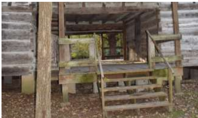
Figure 7: Mold around dimensional lumber on back porch.
