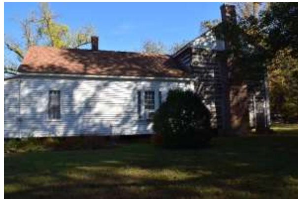
Figure 29: Trim grass/garden away from ell. Keep bush trimmed to allow airflow.
