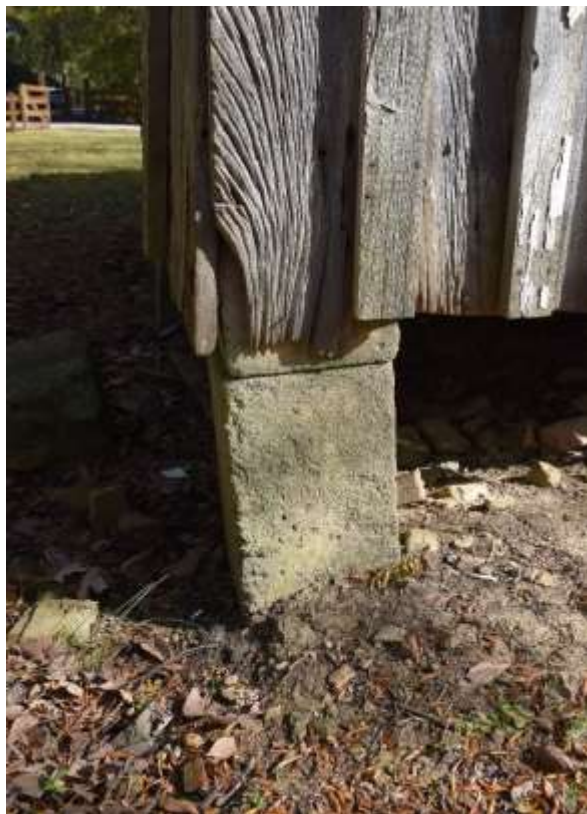
Figure 8: Leaning corner block.
