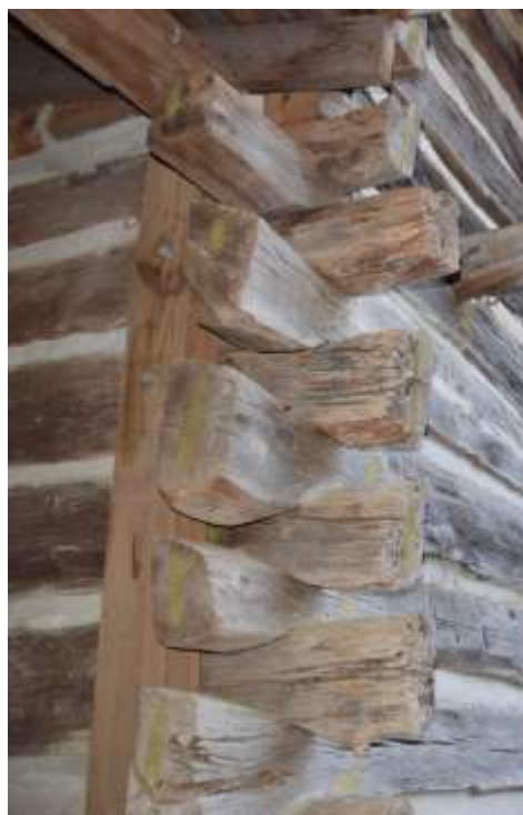
Figure 8: Decayed ends of logs.
