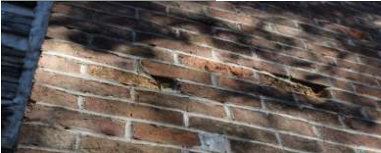
Figure 26: Mold and stains on north chimney.
