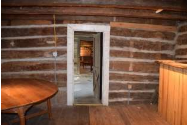
Figure 2: Settling logs on the north wall of the southern room. Possible sign of settling or weakened foundation.
