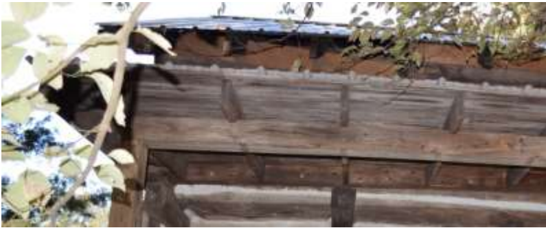
Figure 11: Plywood used to fill the spaces between the rafters is falling, creating access to the loft.
