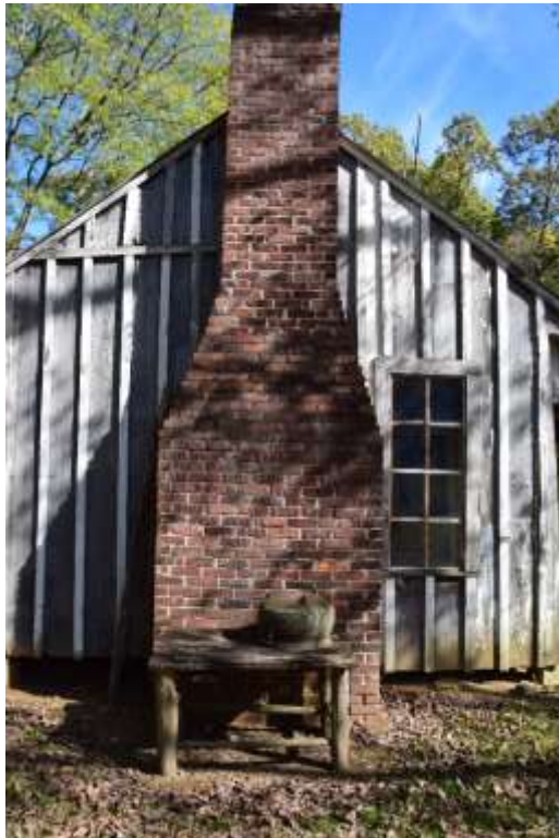
Figure 12: Fireplace chimney showing signs of mortar repair.
