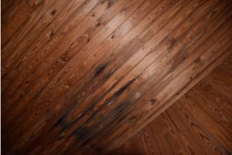
Figure 19: Moisture damage on ceiling. Check for leaks and confirm that mold is not growing above area showing signs of water damage.
