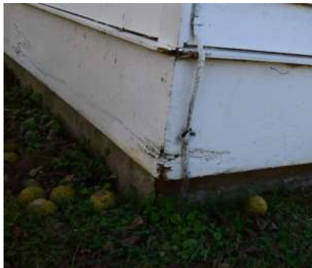
Figure 24: Water damage on skirt board on bathroom addition.
