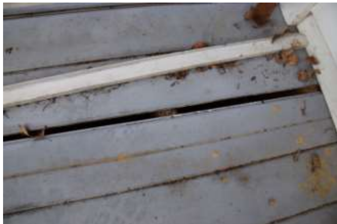
Figure 20: Gaps from expansion and contraction due to improper material.
