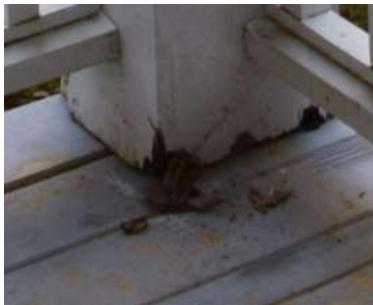
Figure 21: Decay at the base of post due to improper caulking and floor movement.
