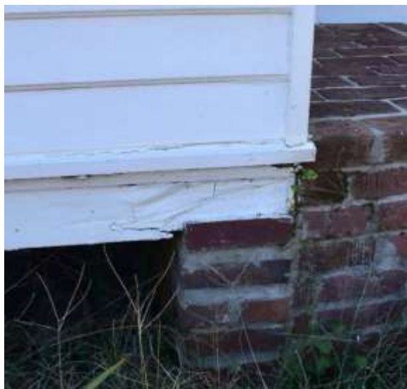
Figure 23: Water damage on skirt board on kitchen extension.
