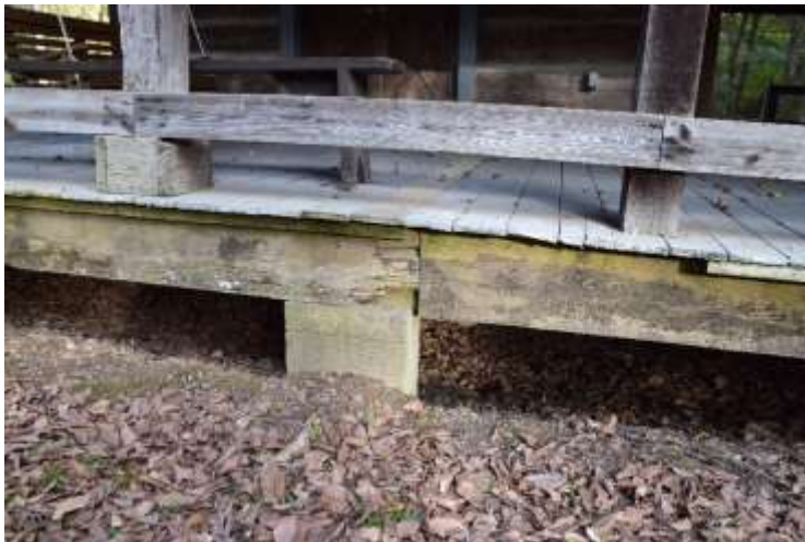
Figure 3: Rotted rim board and loose leaves under front porch.
