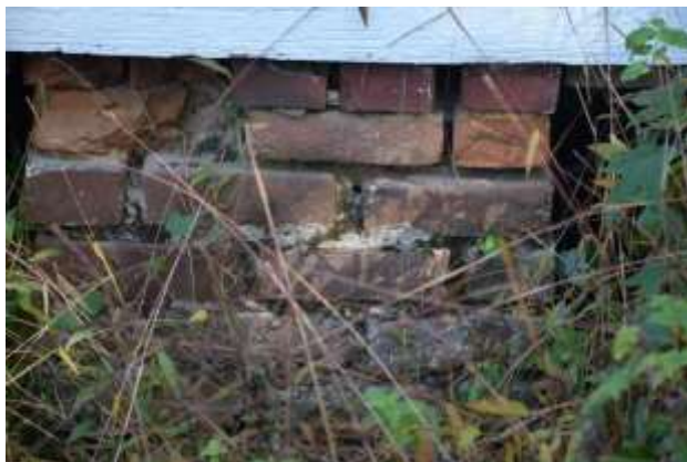
Figure 22: Broken brick and missing mortar on pier.
