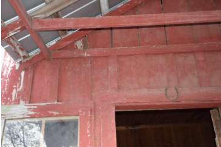
Figure 17: Missing batten under front porch and decay from possible leak where porch cover meets the gable-end wall.
