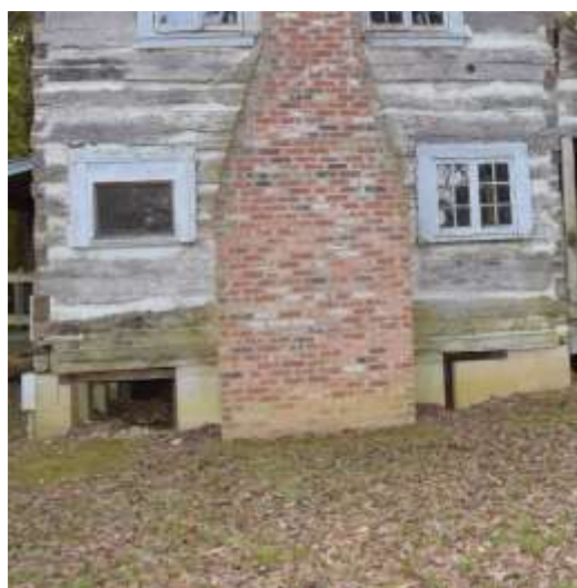
Figure 8: Mold on lower portion of north wall and angles of brickwork on chimney.
