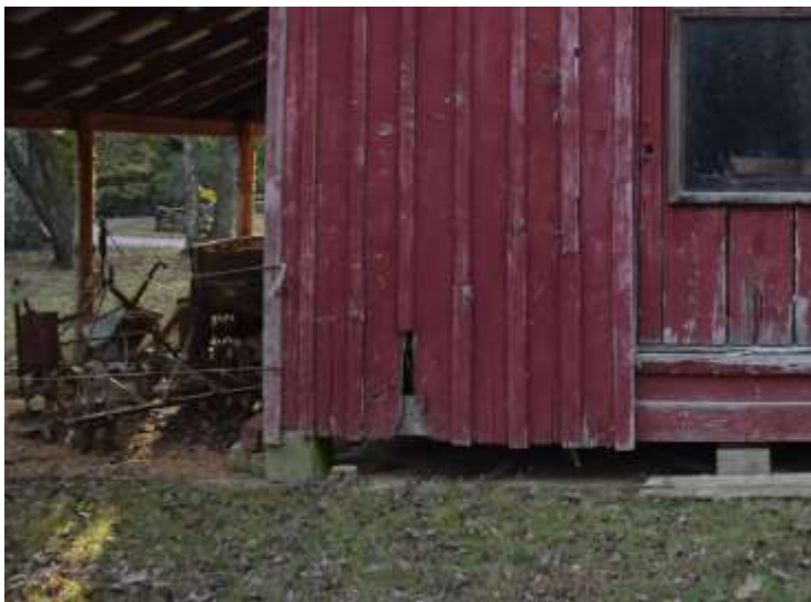
Figure 18: Missing batten on rear of building.
