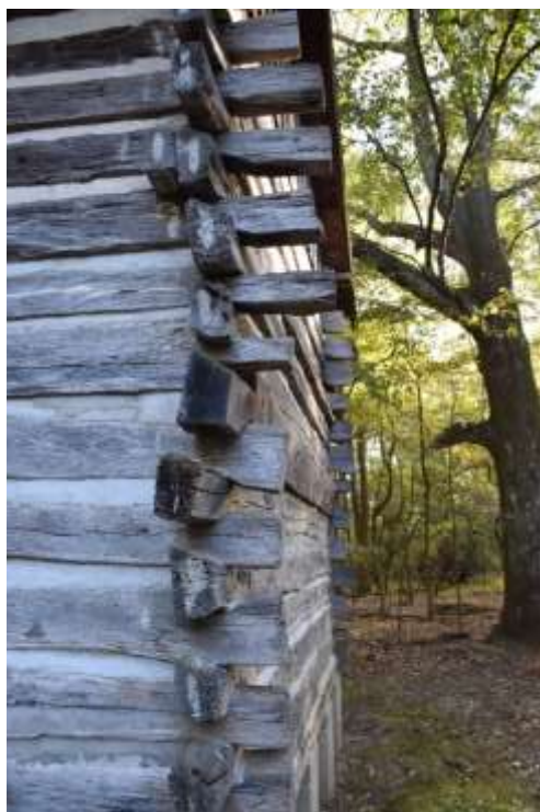
Figure 7: Broken notch causing log to twist out of place.
