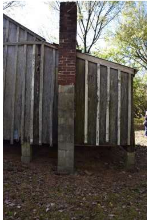
Figure 13: Flue chimney for stove showing signs of mortar repair and stabilization.
