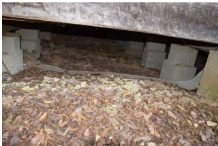
Figure 5: Loose leaves and materials under floor should be removed to reduce moisture and decrease the likelihood of invasive species.
