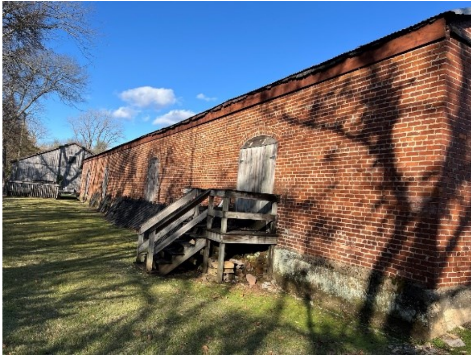
West Elevation: Mold on Foundation, Worn Stairs, Missing Gutters on Roof
