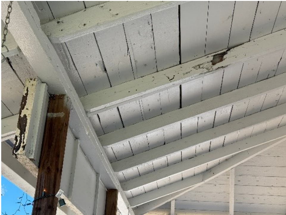
Rotted Beams for Front Porch Roof
