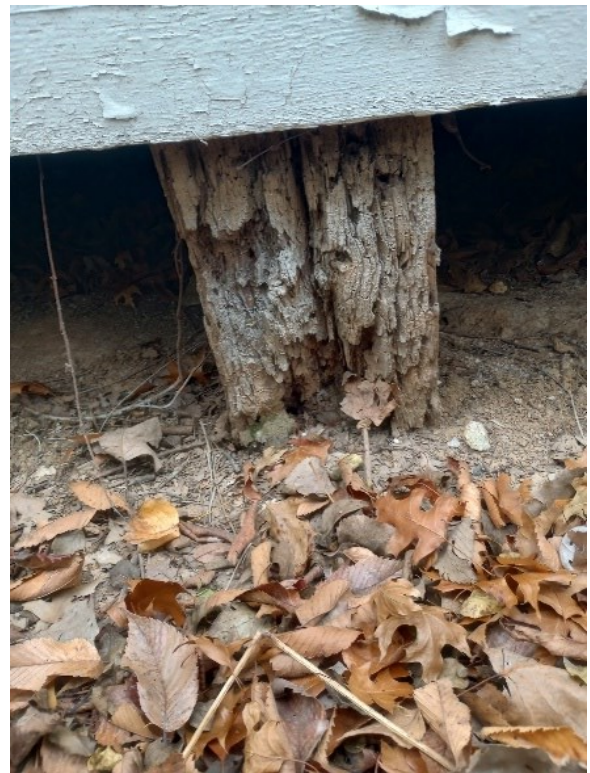
Damaged Wood Foundation Block
