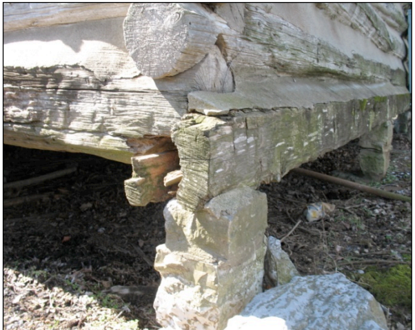
Sill at Schoolhouse needs replacement.
