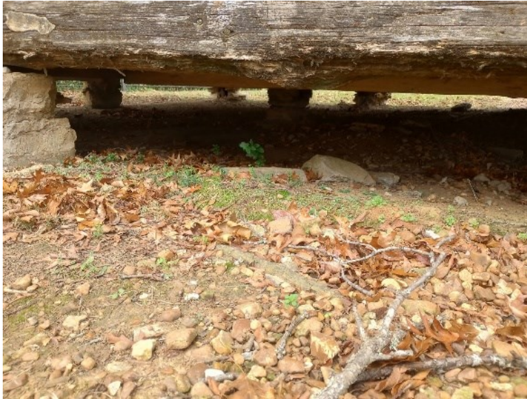
East Elevation: Drainage Issue Under Building
