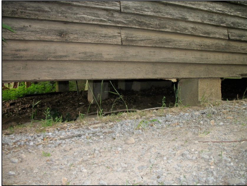
Depression under building attracts water and holds moisture.
