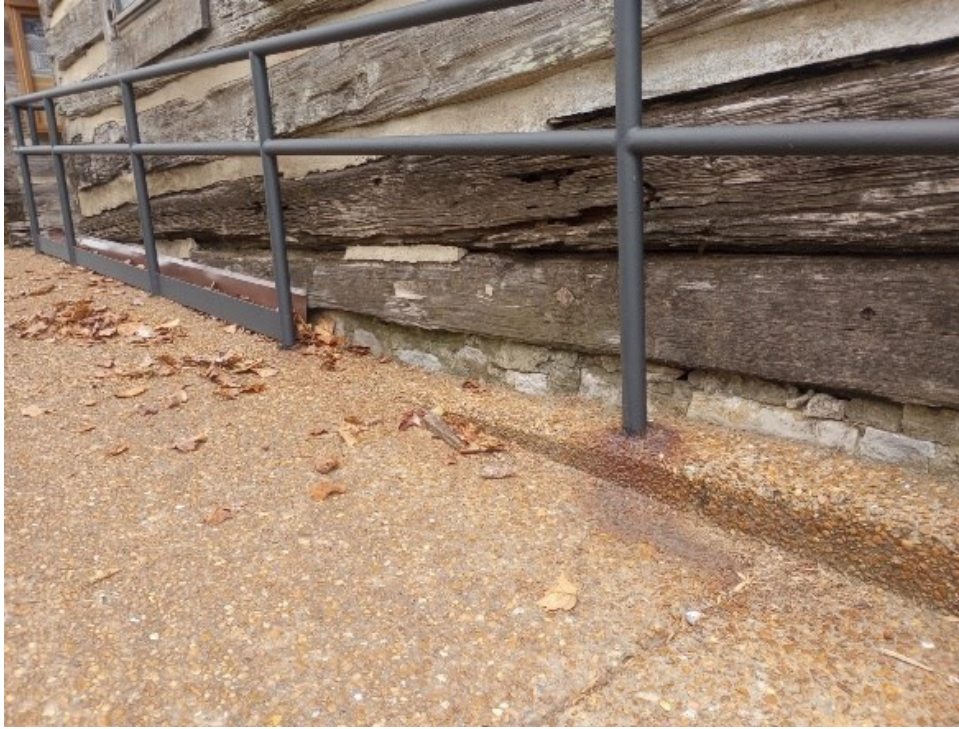
Northwest Elevation: Chinking and Daubing Damage
