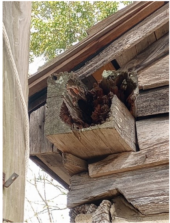
Southwest Elevation: Rotted Logs
