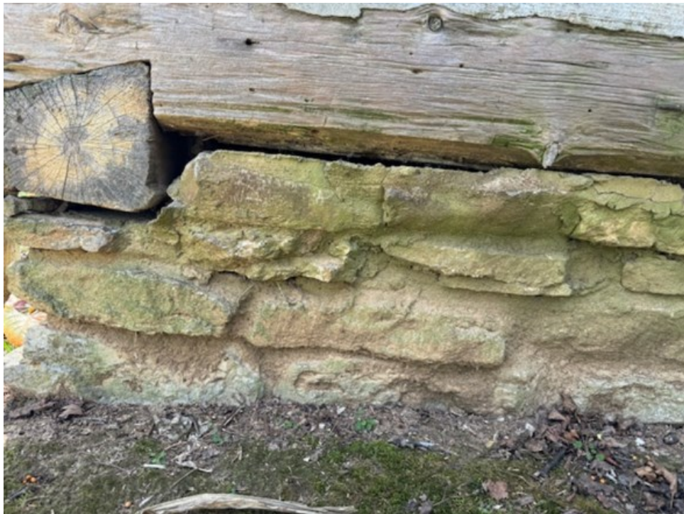
Gaps Between Wood and Foundation West Elevation
