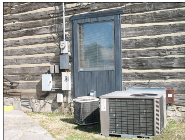
Electrical boxes and HVAC unit at Visitor Center
