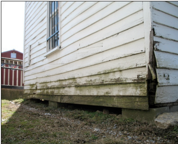
Doctor’s Office mold and siding deterioration
