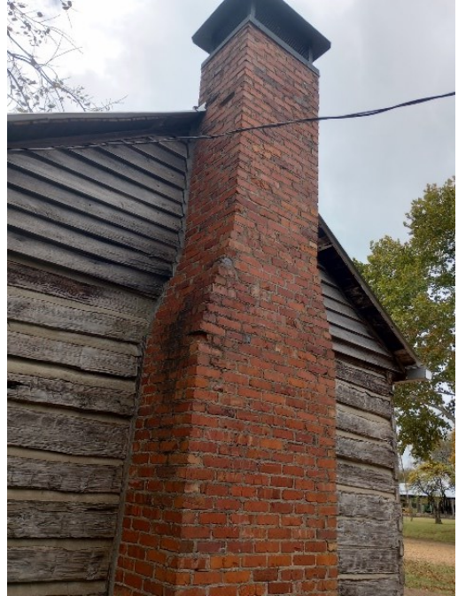
West Elevation: Damaged Chimney
