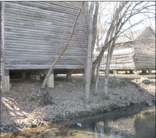
Grist mill foundation endangered by erosion.
