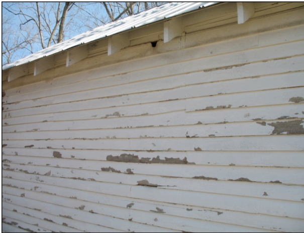
General Store paint failure
