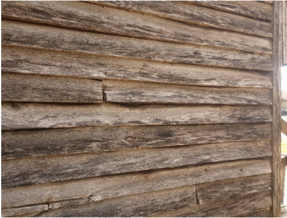
East Elevation: Damaged Siding
