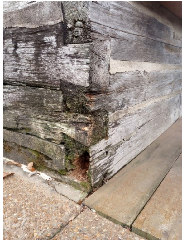
Northwest Elevation: Rotted Logs with Mold and Moss Growth
