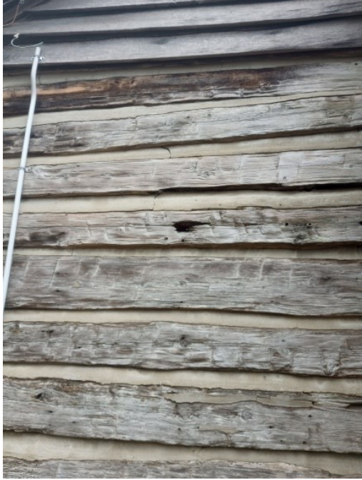
West Elevation: Damaged Siding
