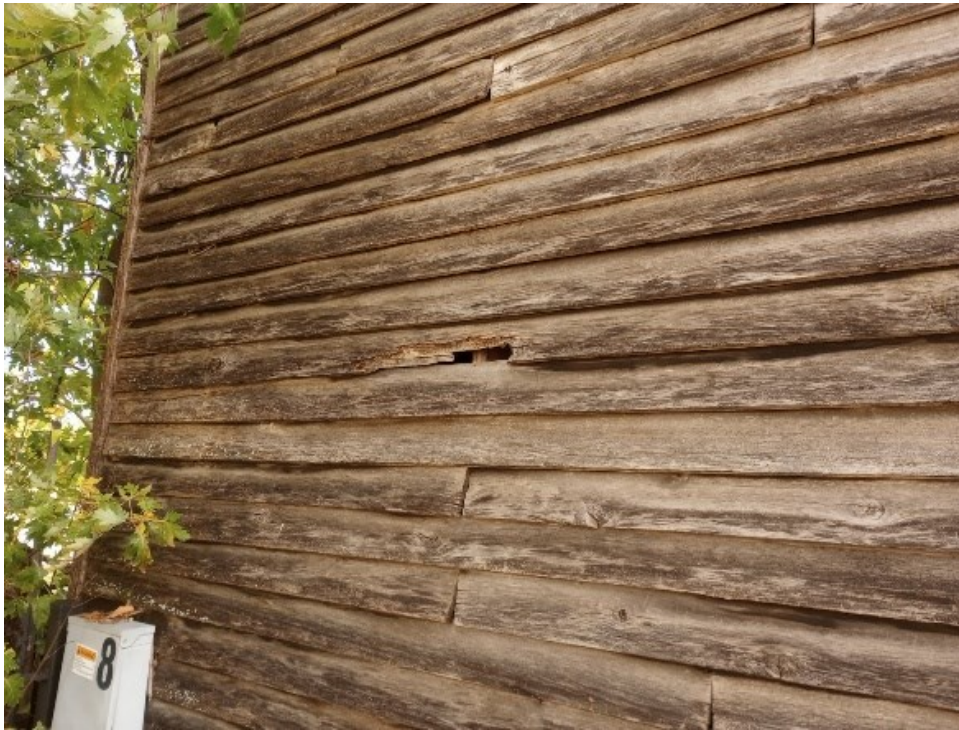
West Elevation: Damaged Siding
