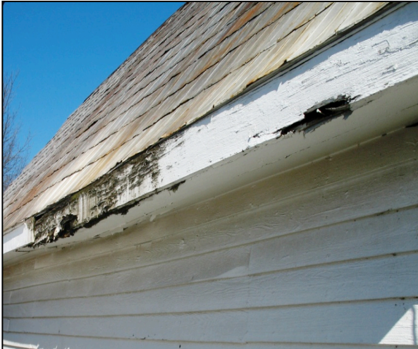
General Store cornice deterioration
