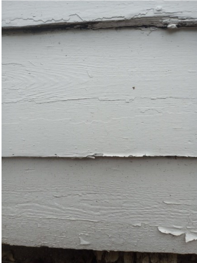
West Elevation: Peeling and Chipping Paint
