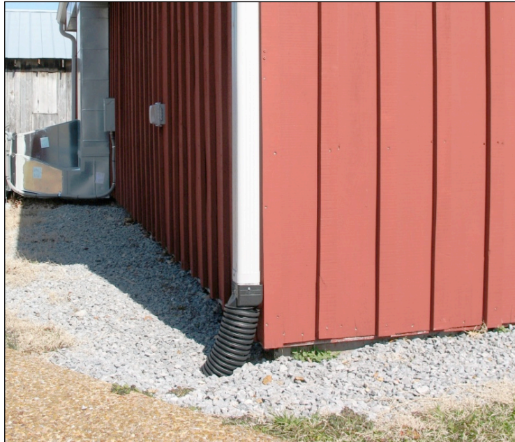
Gutter system at the Stones River Garage drains rainwater.
