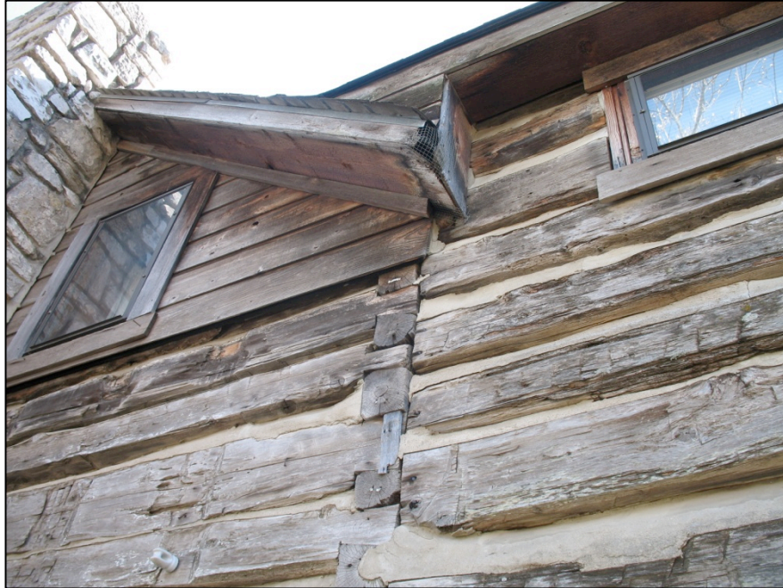
Wooden trim deterioration at Visitor Center needs to be repaired.
