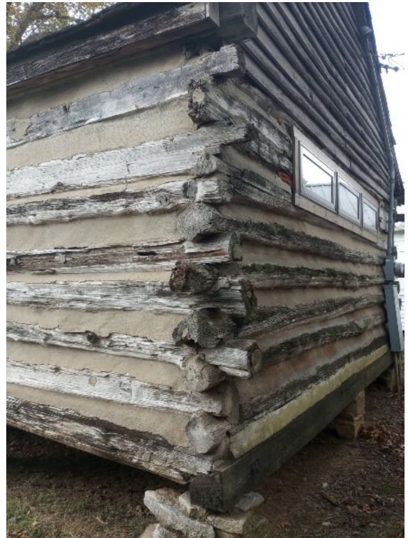
Northwest Elevation: Rotted Logs
