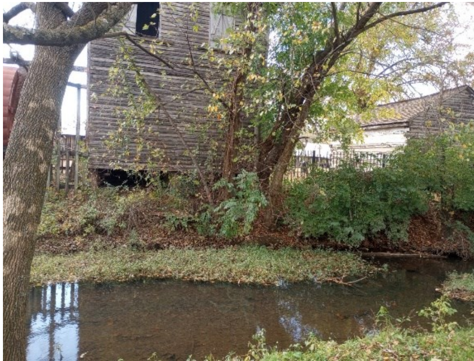
North Elevation: Missing Window Shutter
