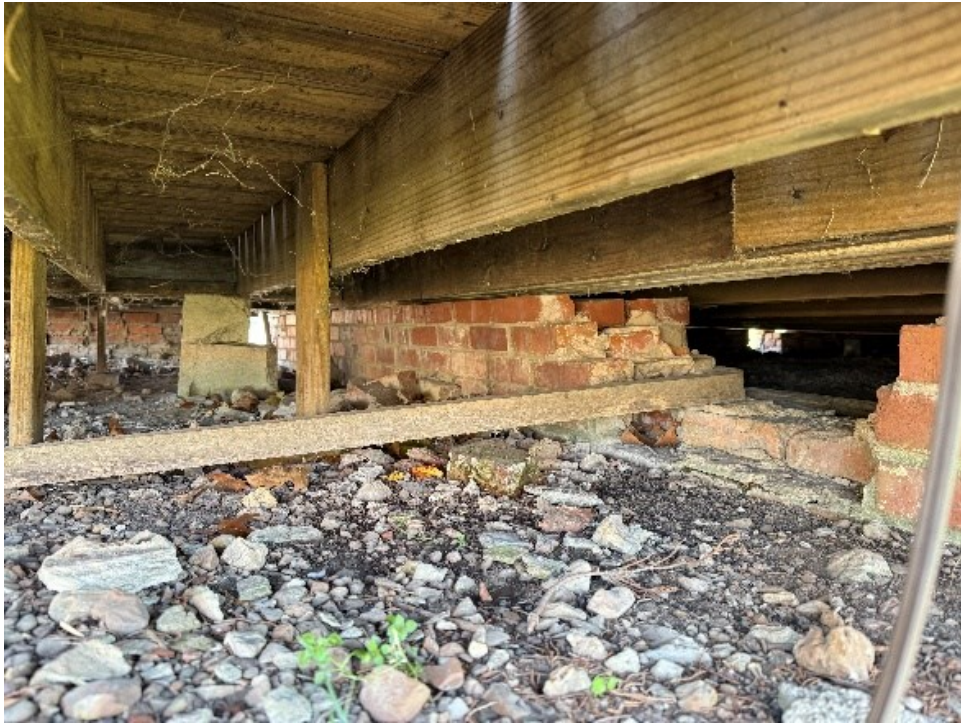
Lack of Moisture Barrier Beneath General Store
