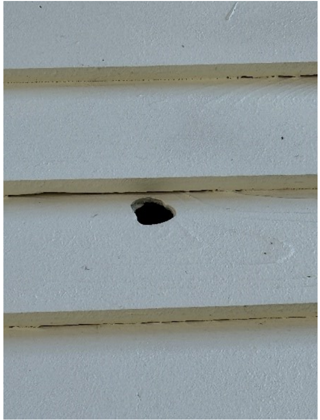
Hole in Siding
