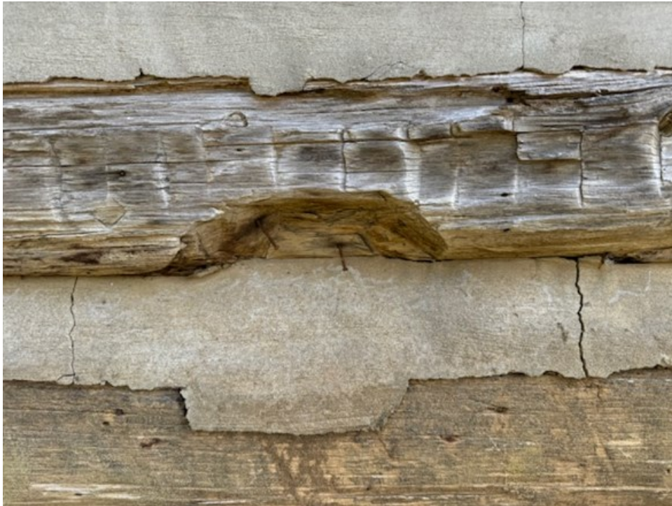
Wood Missing West Elevation
