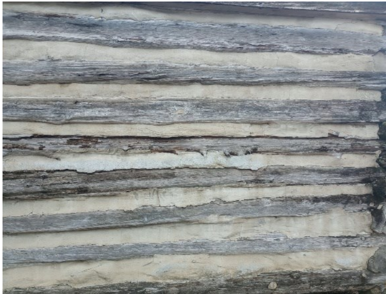
West Elevation: Chinking and Daubing Damage
