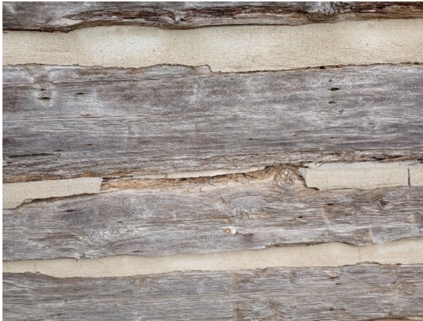
Chinking and Daubing Damage
