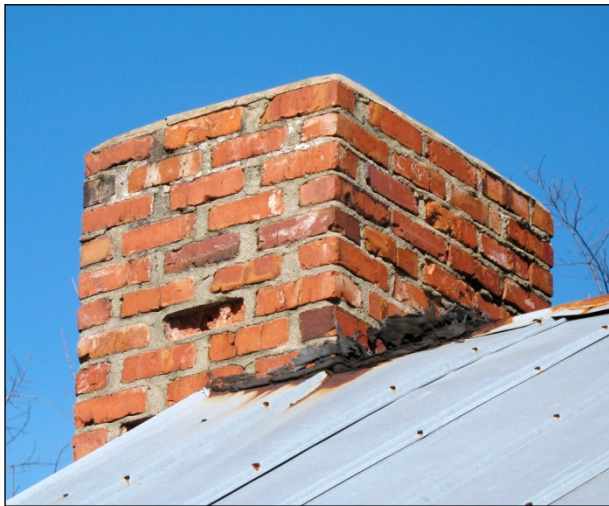
Inadequate tar flashing on University House.
