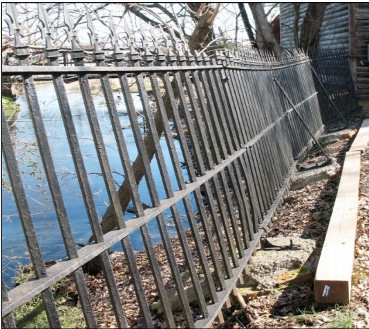
Iron fence footings undercut by flood waters.
