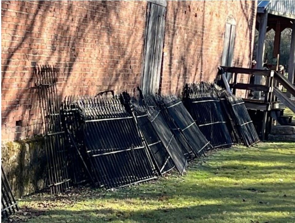
West Elevation: Unsafe Wrought Iron Fencing
