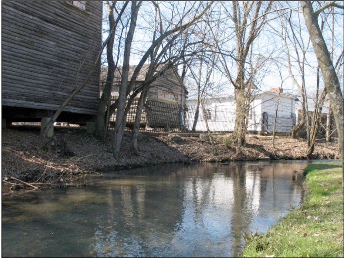
Town Creek bank erosion undercuts foundations.
