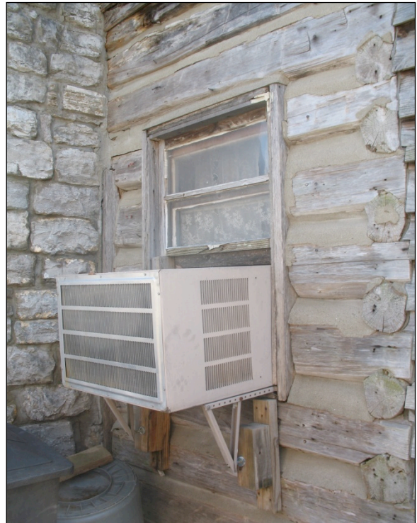
Window air conditioner at Leeman House
