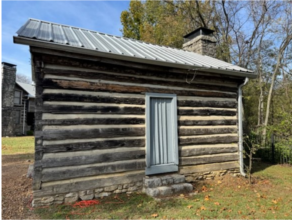
Side Door, Exposed Wiring, and Rain Gutter System East Elevation
