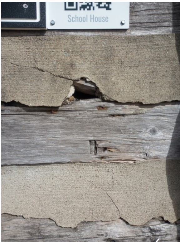
Southwest Elevation: Chinking Damage
