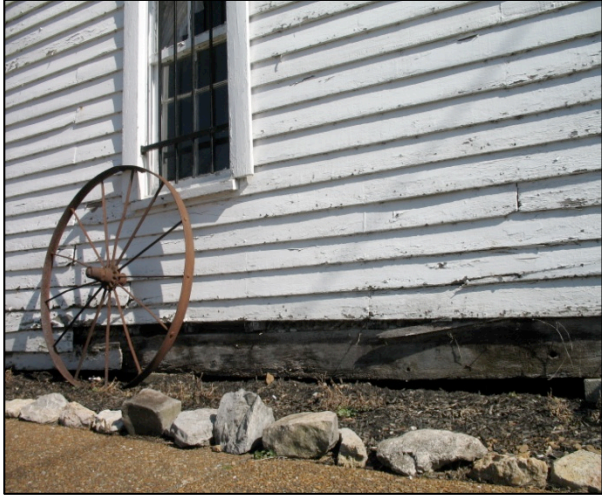
Mold on Doctor's Office foundation.
