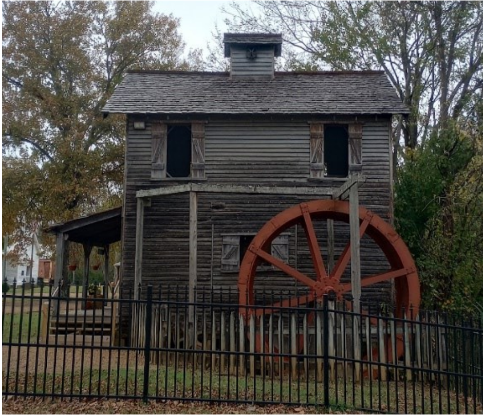
East Elevation: Mold Growth
