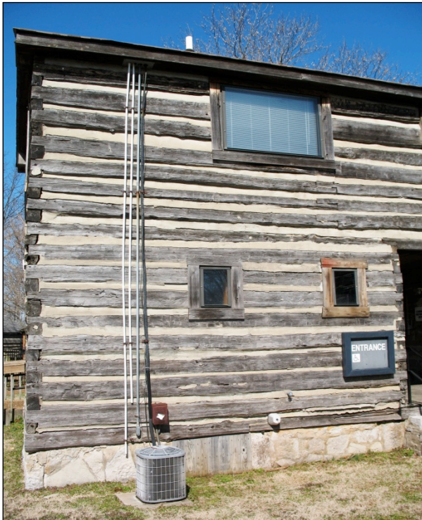
HVAC unit at Visitor Center
