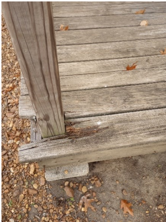
South Elevation: Damaged Front Porch
