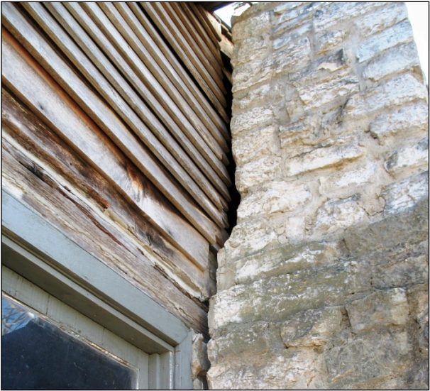
Town Hall gable siding voids
