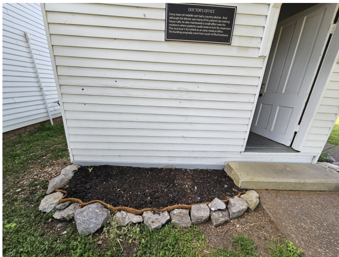
Mulch Close to Foundation
