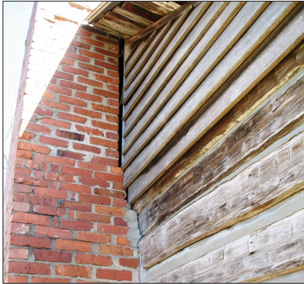
University House gable siding voids
