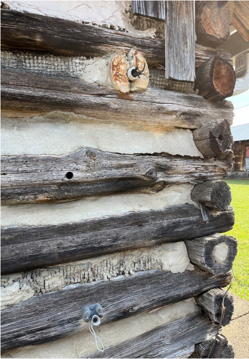
Degraded chinking and daubing West Elevation
