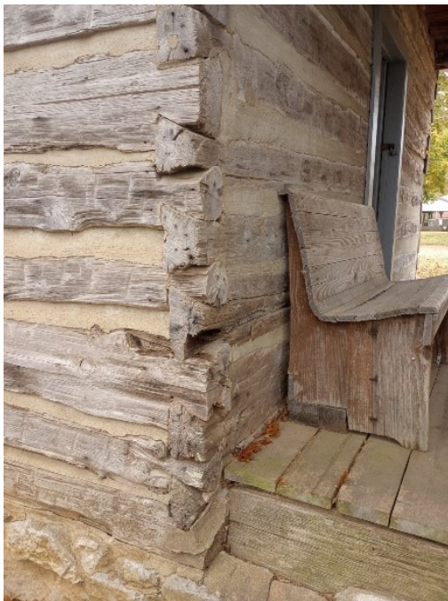
North Elevation: Rotted Logs
