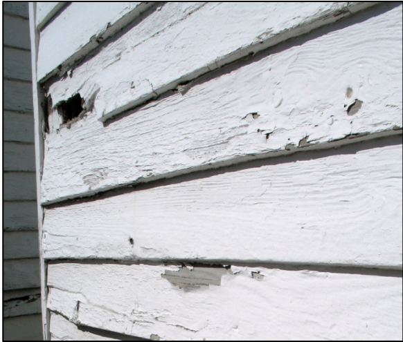
Doctor’s Office siding and paint deterioration
