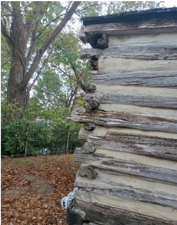
Northwest Elevation: Rotted Logs
