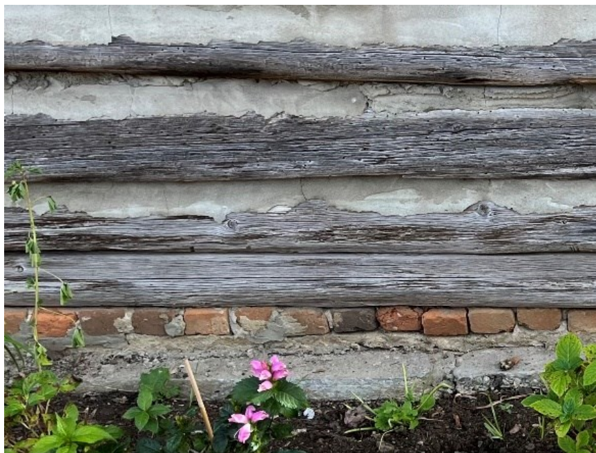
Brick Foundation with Missing Mortar West Elevation
