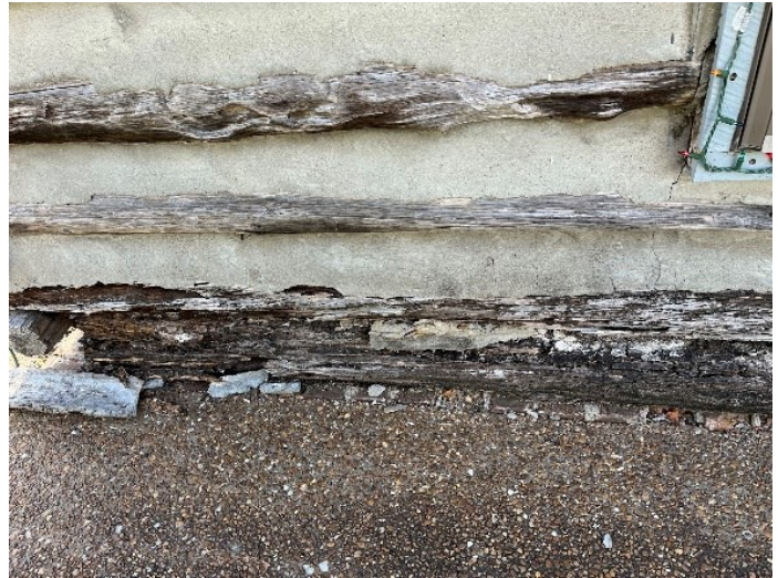
Degraded logs North Elevation
