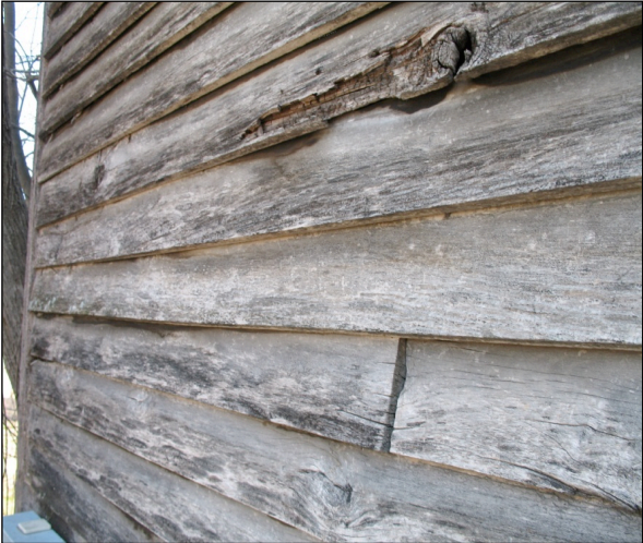
Grist Mill siding deterioration
