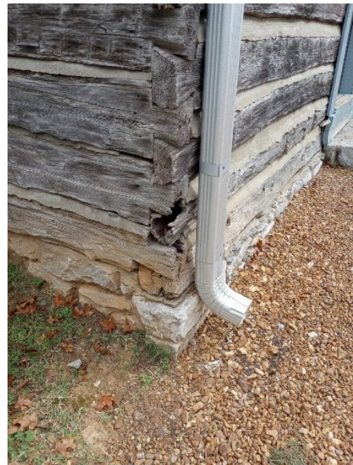
East Elevation: Chinking and Daubing Damage
