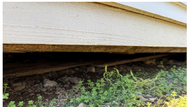
Lack of Moisture Barrier Beneath Structure
