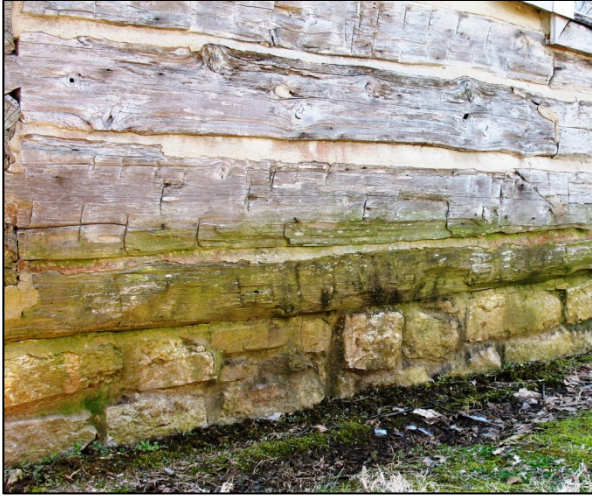
Moss and mold on University House foundation.
