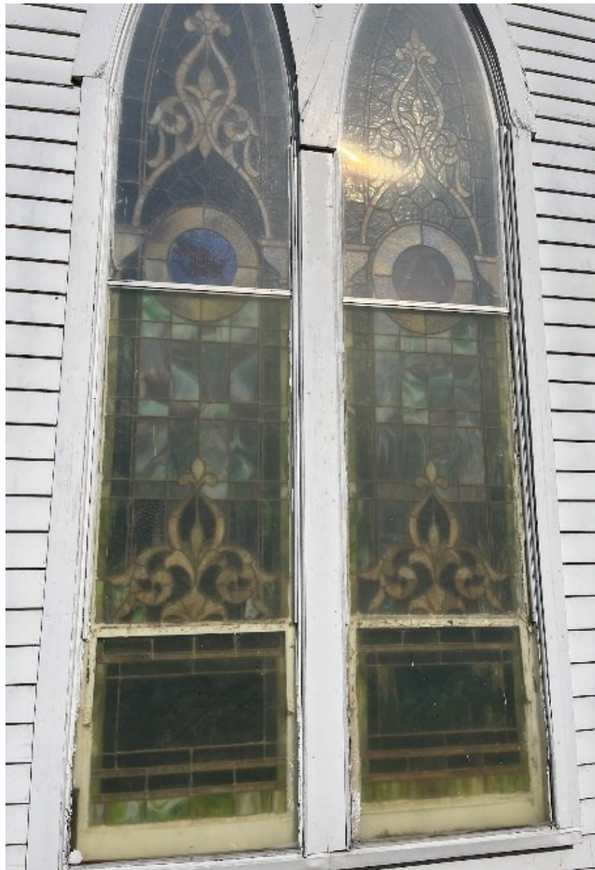
Windows in Disrepair South Elevation
