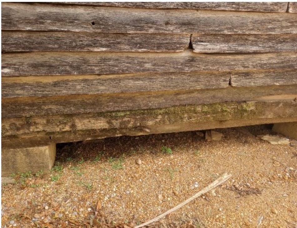
West Elevation: Damaged Siding
