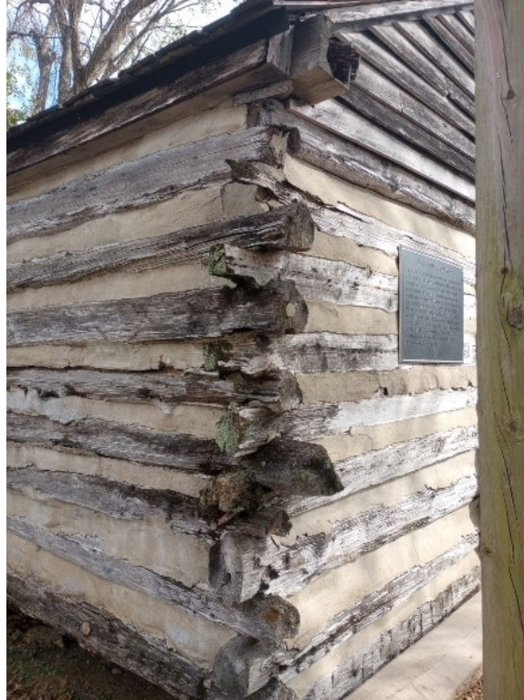
Southwest Elevation: Rotted Logs
