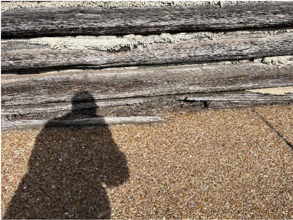
Degraded Logs South Elevation
