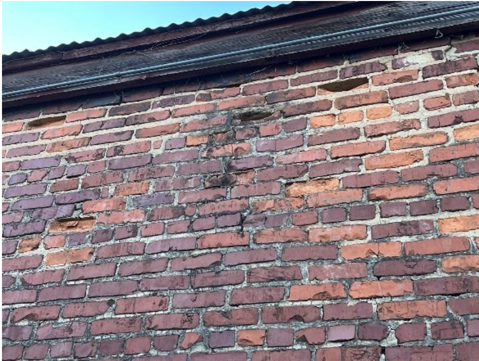
Roof East Elevation (No Gutters), Damaged Bricks, Damaged Roof Line
