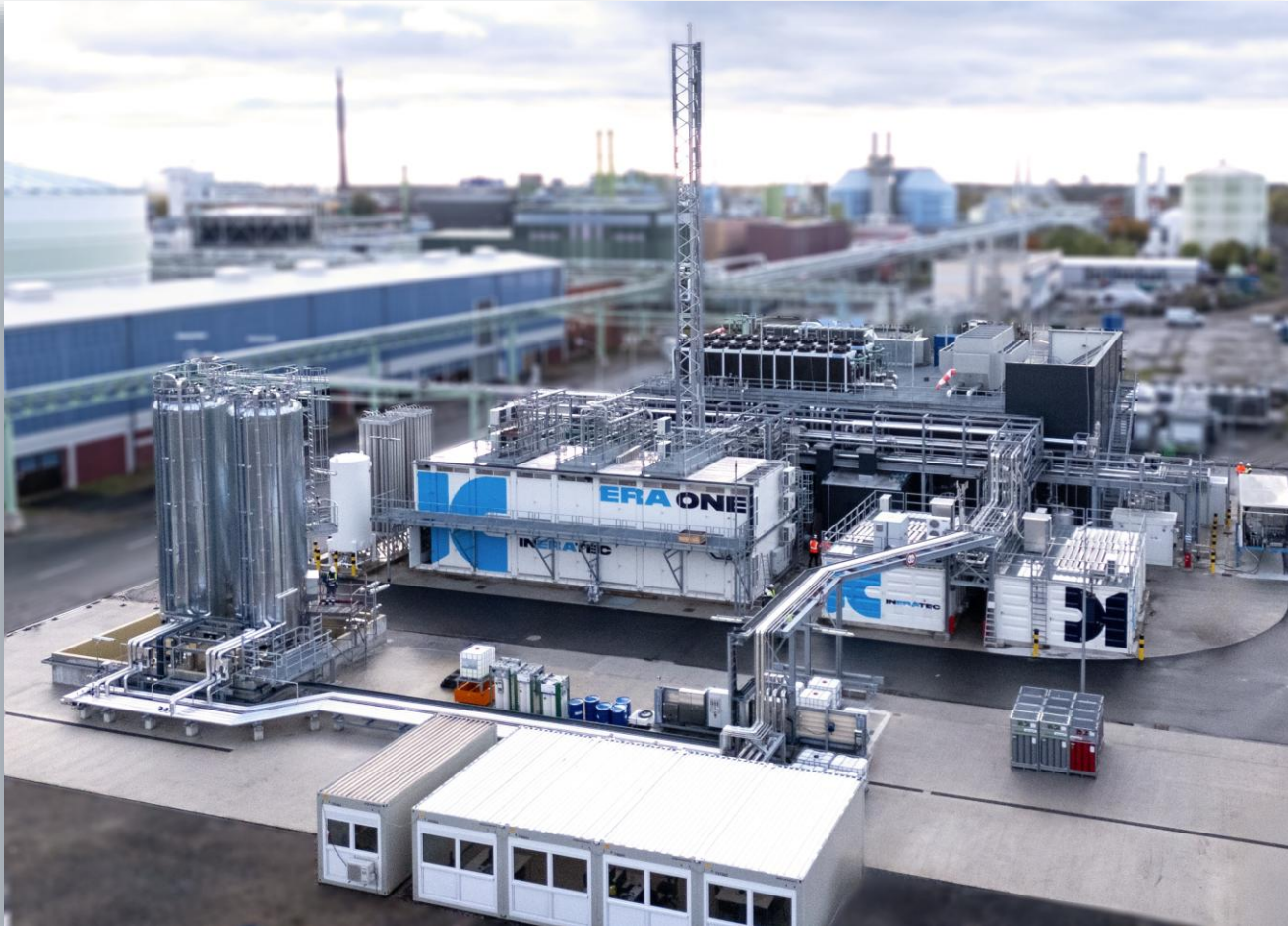
Photo Credit: INERATEC's ERA ONE Pioneer Power-to-Liquid plant at Frankfurt Höchst © INERATEC GmbH 2026
