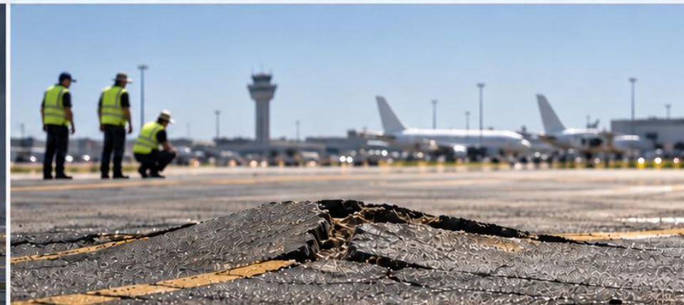
LUTON — RUNWAY HEAT DAMAGE
