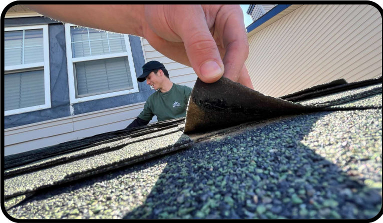
Cracking or Splitting
