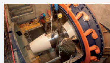
Bulb unit: Dismantling of old unit and erection of new one. Weinzödl HPP, Austria; 8,66 MW, 2 units
