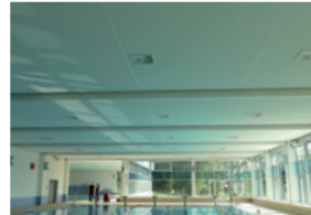
Tensioned ceiling - Aqua centre (CH)
