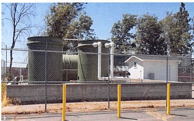
Figure 1: This 20,000 gpd Bio-Pure wastewater treatment system was installed in 2003 in the City of Paradise, California. Except for a brief period in 2018 when the small building that houses the operating system and electrical panels was destroyed by a fire, this unit has been operating successfully since its installation. It processes wastewater from a large shopping center in the commercial area of the city. The clean effluent is discharged to a leach field beneath the asphalt parking lot of the shopping center.
