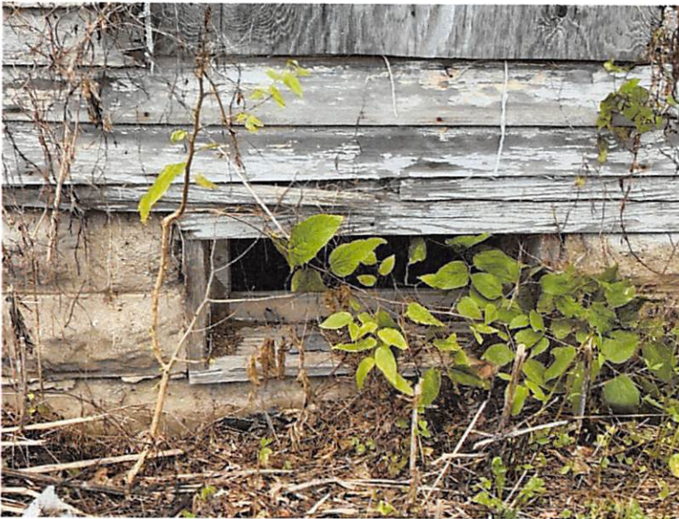
Small window at base of foundation – window missing
