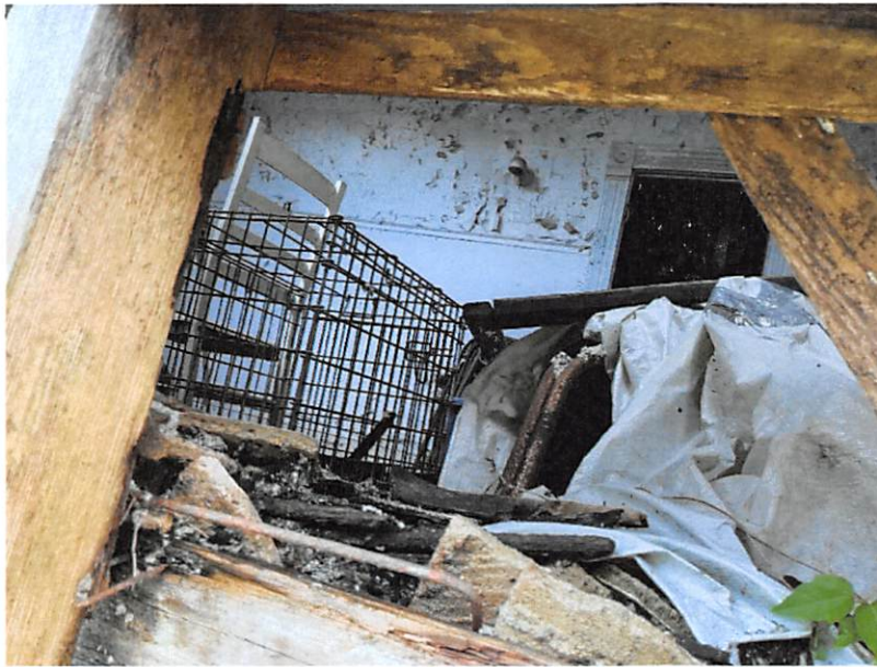
Hole in wall of dwelling
