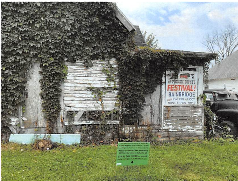
View of dwelling from Indiana Avenue – shows missing siding and holes in structure
