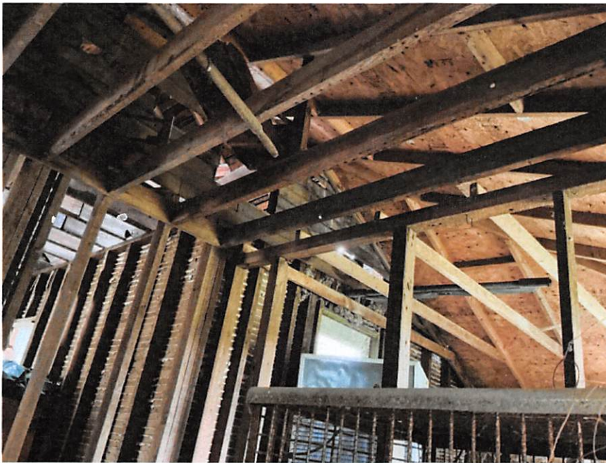
Look at the rafter showing daylight
