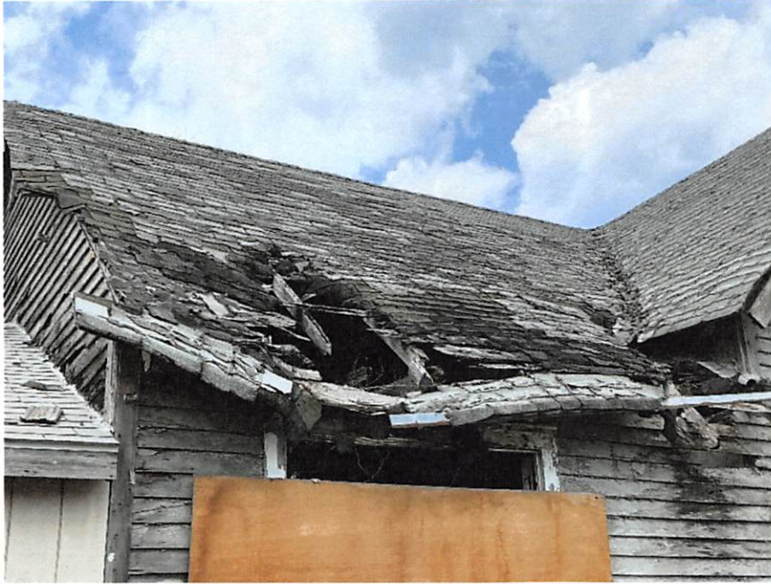
Roof falling in; windows partly boarded – window missing
