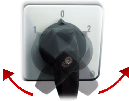
Figure 4. Main Control Switch
