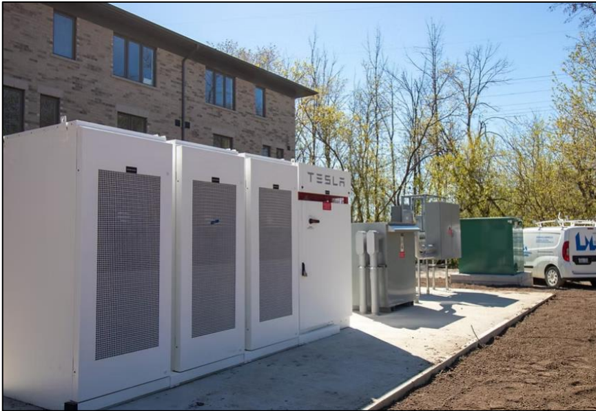
Altona Towns (250 kW / 500kWh). Construction completed 2021.
