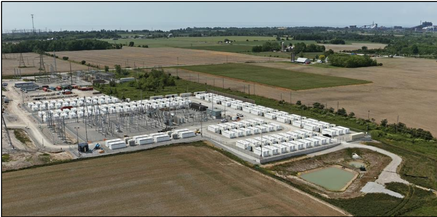
Oneida BESS (250 MW / 1,000 MWh), Haldimand County. Operational since May 2025.
