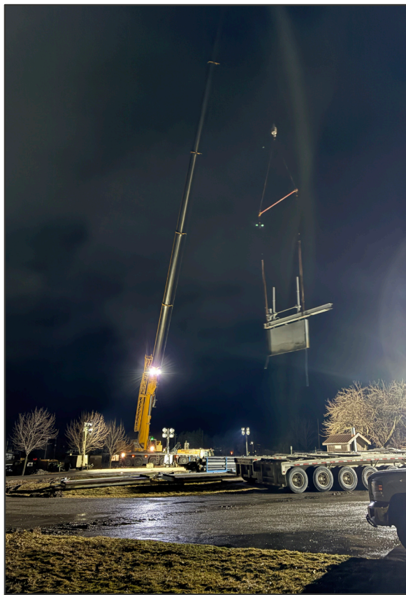
A crane company was brought in Sunday night to remove the gates from the Cheboygan Dam to increase the water flow.
