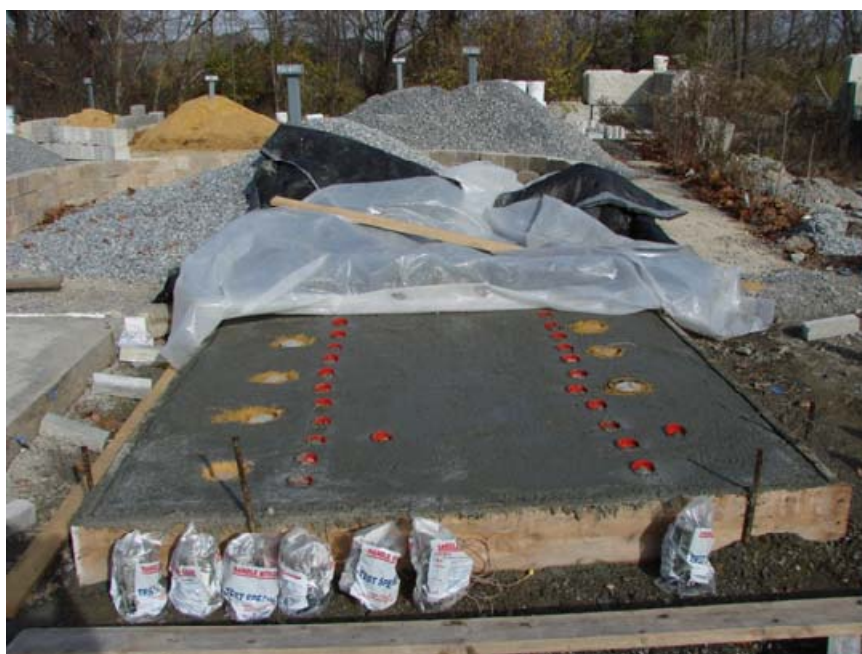
Figure 4.8 Slabs with cast-in-place cylinders, floating inserts and field cure cylinders (The red marking are the pullout inserts, field-cured cylinders are placed outside the slab and the cast-in-place cylinders are within the slab)
