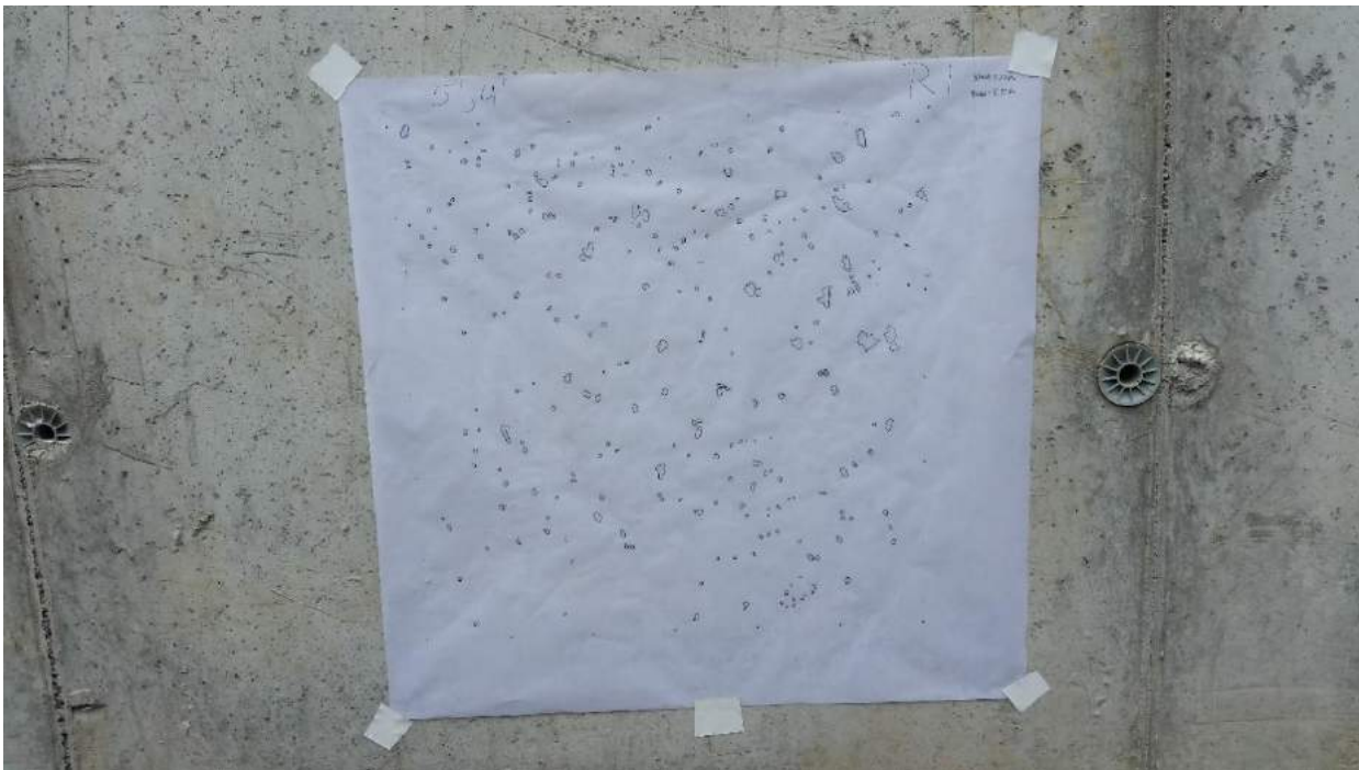
Fig. 6.14 Cast-in-place wall being measured by NJIT student researchers on active construction site
