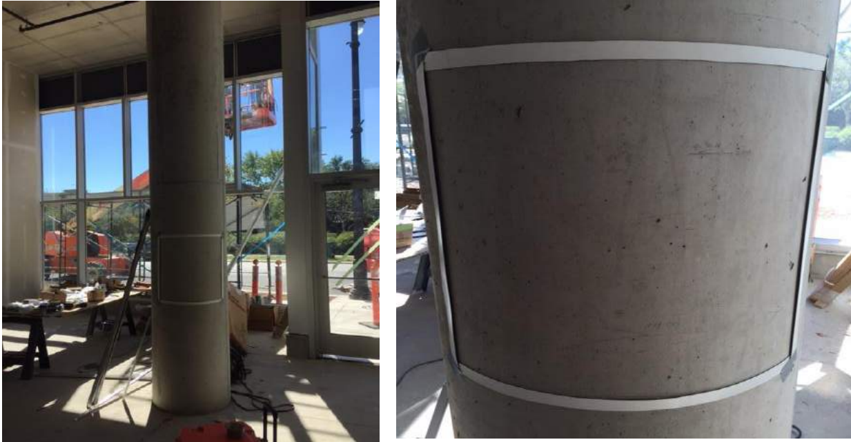
Fig. 6.19 Lab B circular column viewed from 20 ft and close-up of the sampled area. SVR for one sample = 0.4%.
