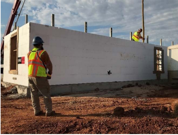
Image 3: Pump truck operator and foreman working in tandem to place concrete inside ICF walls
