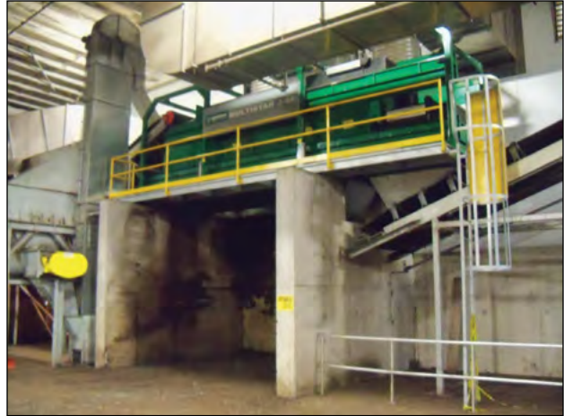
Photo 9-5: Designers should provide appropriate ladders and catwalks so equipment can be easily accessed for inspections and maintenance © CH2M HILL
