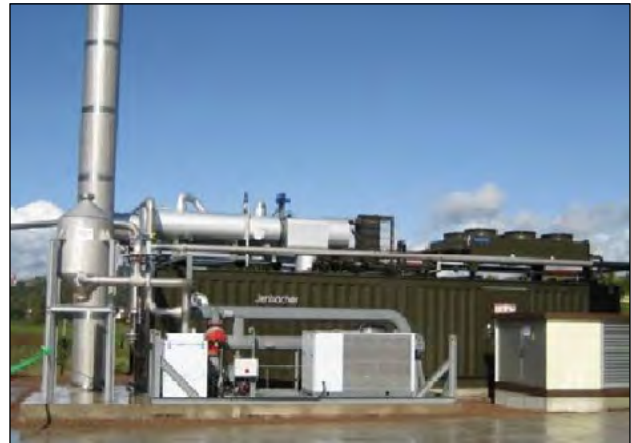
Photo 7-1: Package CHP system © CH2M HILL
