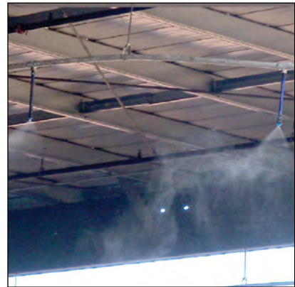
Photo 15-2: Roof-mounted and directional misting systems installed inside buildings and around equipment are effective at controlling dust levels © CH2M HILL
