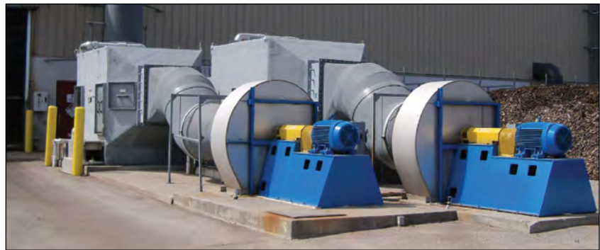
Photo 14-5: Atomized mist scrubber © CH2M HILL
