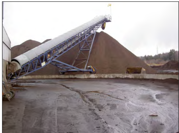
Photo 11-17: Radial stacking conveyor © Scott Gamble
