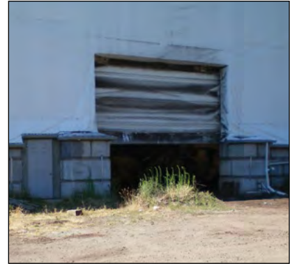
Photo 9-7: Leaving doors open impairs the ability of a building's ventilation systems to contain odours © CH2M HILL
