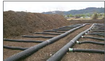
Photo 5-11: Outdoor composting piles with a pipe-on-grade system © CH2M HILL
