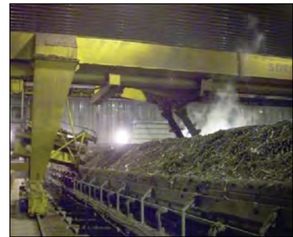
Photo 5-27: Bridge crane and suspended auger turning mechanism viewed from discharge side of bay © Scott Gamble
