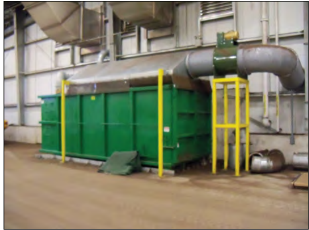
Photo 10-7: Enclosed roll-off containers can be used to contain litter and residuals from preprocessing and screening operations © CH2M HILL
