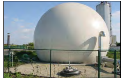
Photo 4-1: Biogas storage tank © Organic Waste Systems Inc.
