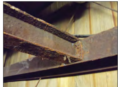
Photo 9-12: Corrosion has proven to be one of the most challenging design issues for the organic processing industry © CH2M HILL
