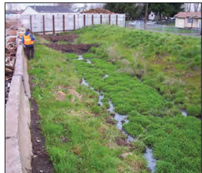
Photo 10-10: Filter berms and bioswales can be a cost-effective way to remove sediments from uncontaminated stormwater © Scott Gamble
