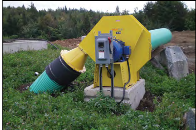
Photo 8-3: Aeration fans used at composting facilities normally require three-phase power supply © CH2M HILL
