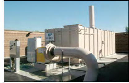
Photo 14-8: Enclosed biofilter system at a composting facility © Biorem Technologies Inc.
